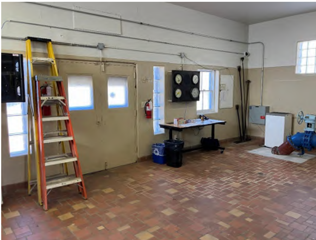
Interior of existing Wellhouse.
