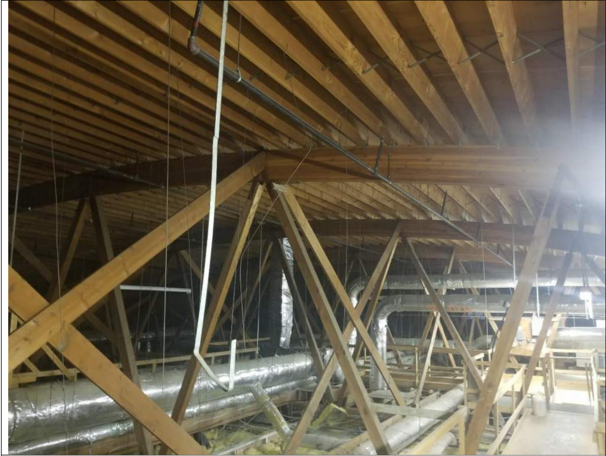
INTERIOR MEZZANINE EQUIPMENT FLOOR
