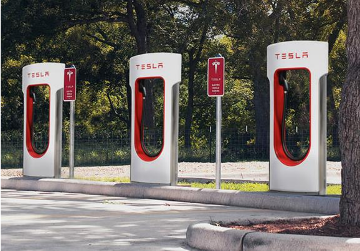
Tesla charging stations
