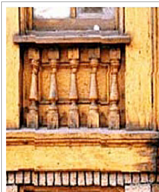
FIGURE 18.4 Wood features on historic properties. Sometimes they can be stabilized instead of stripped of traditional painted finish as in this photo. Photo courtesy of National Park Service.
