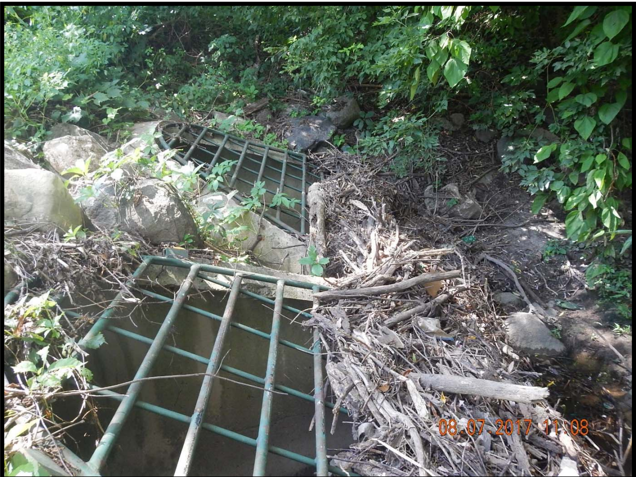
Figure 4: Outlet grates clogged with debris exemplify why access road is needed and why silver maples are often removed from greenway systems.
