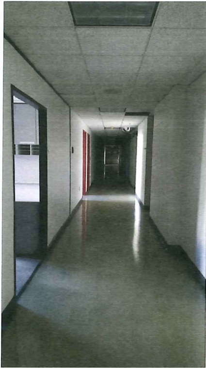
Upper Level Corridor showing asbestos tile
