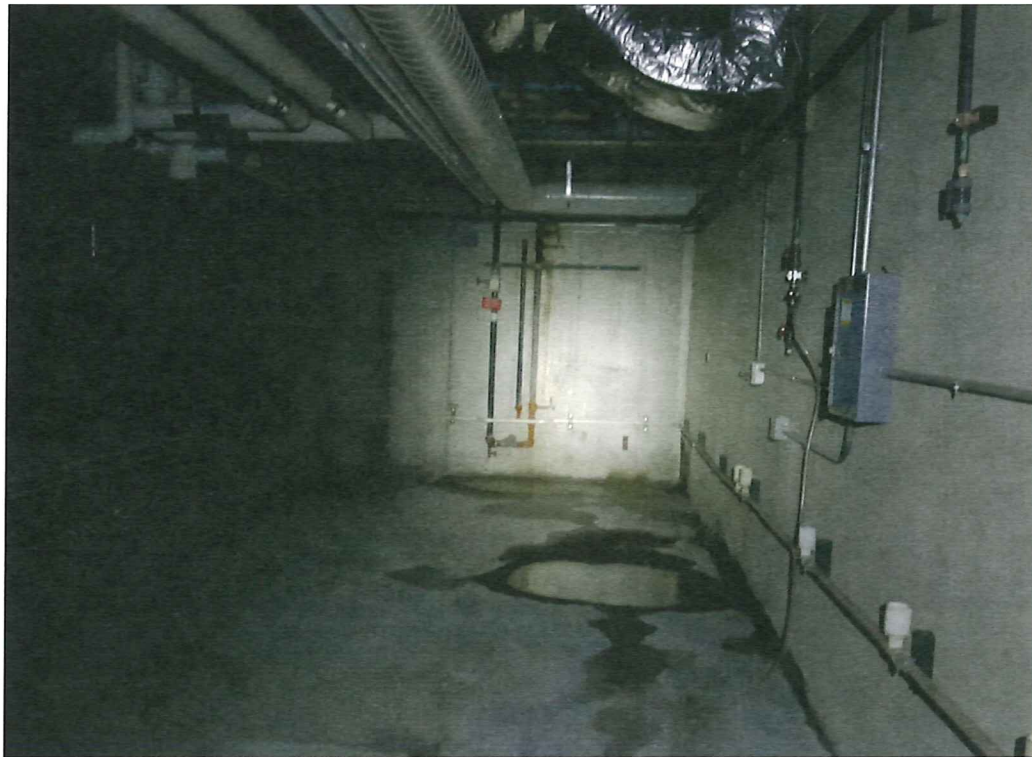
Lower Level Mechanical Space
