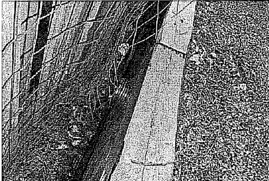
South property line looking towards lake (View of downspout discharge from adjacent property)
