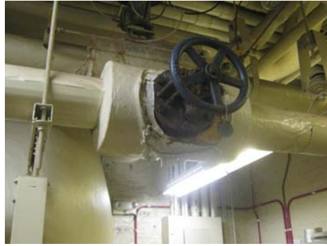
Figure 34 – Leaking Valve and Damaged Insulation
