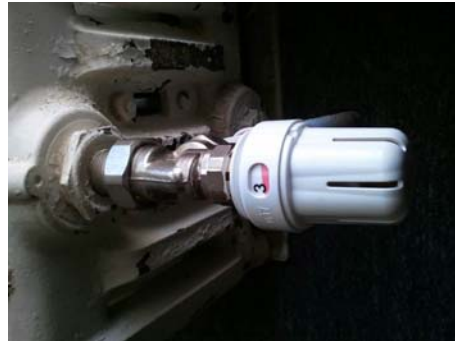
Figure 36 – Steam Radiator Control Valve
