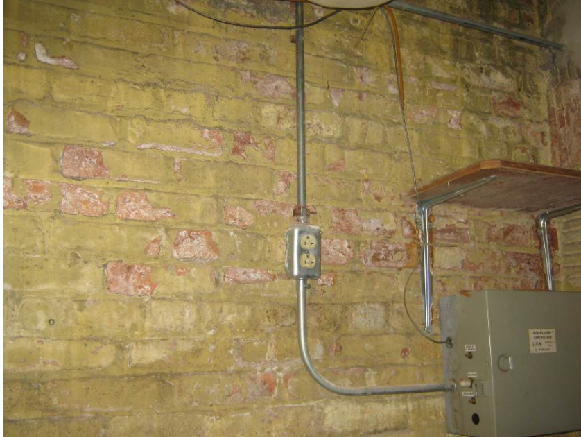
Figure 58 – Existing Brick Basement Wall Water Damage
