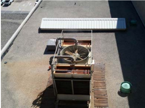
Figure 31 – Cooling Tower Condition
