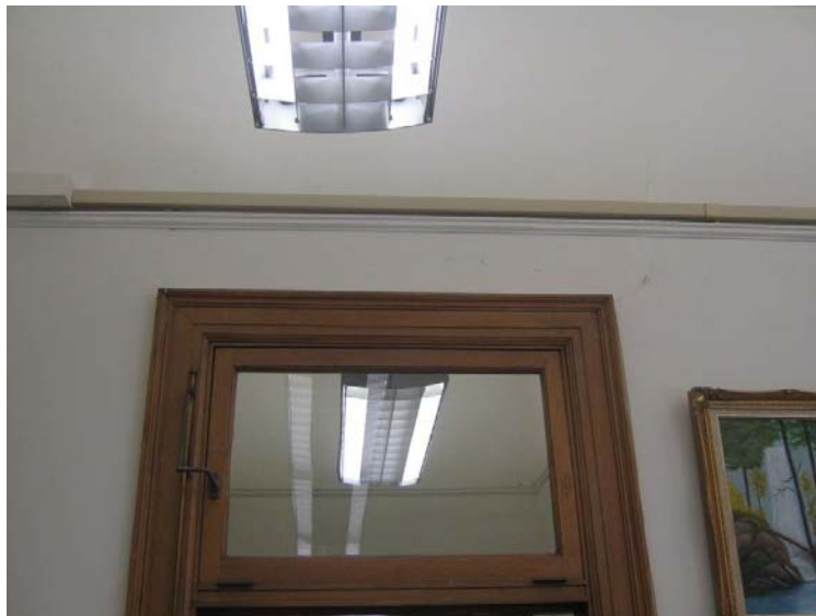
Figure 57 – Plaster Cracking at Corners of Third Floor Door
