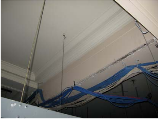
Figure 25 – Original Plaster Ceilings and Decorative Crown Moldings remain above the Suspended Ceilings on the First Floor
