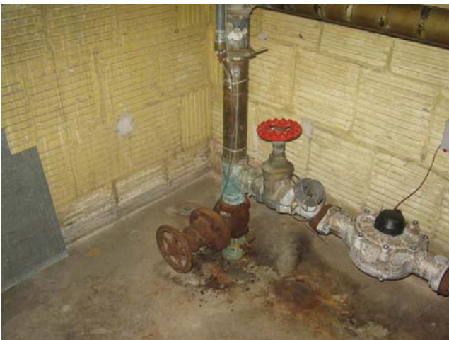
Figure 39 – Incoming Combined Plumbing and Fire Protection Service
