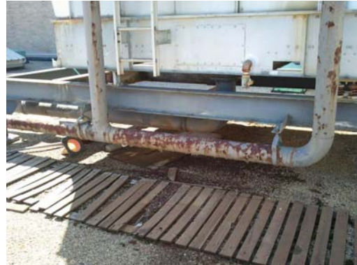
Figure 32 – Cooling Tower Condition
