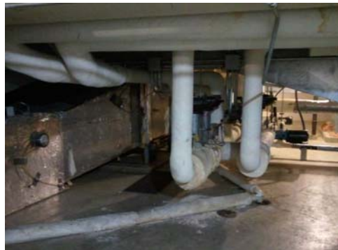
Figure 38 – Ventilation Air Unit for Lower Level and First Floor
