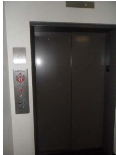
Figure 53 – Elevator Button Interfaces
