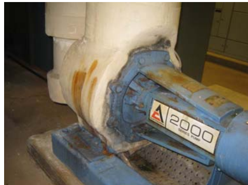
Figure 33 – Rust on Pump Header
