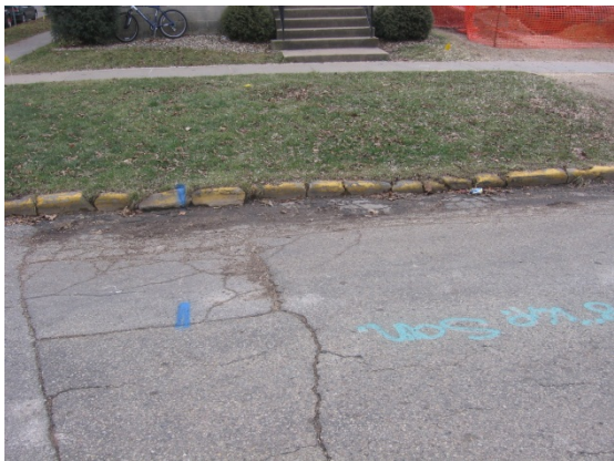
Mound between Orchard and Charter (curb and road in poor condition)
