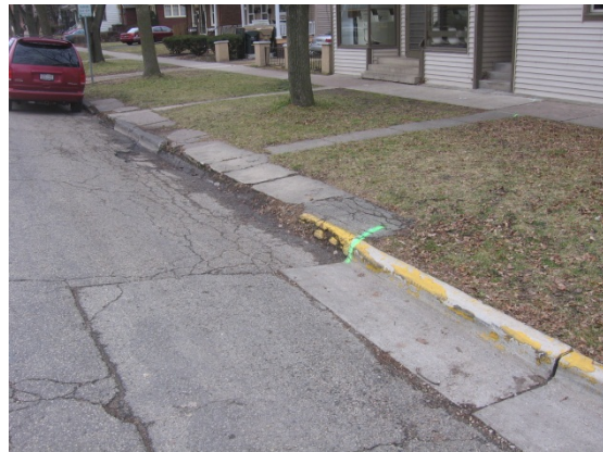
Mound between Orchard and Randall (curb and road in poor condition)
