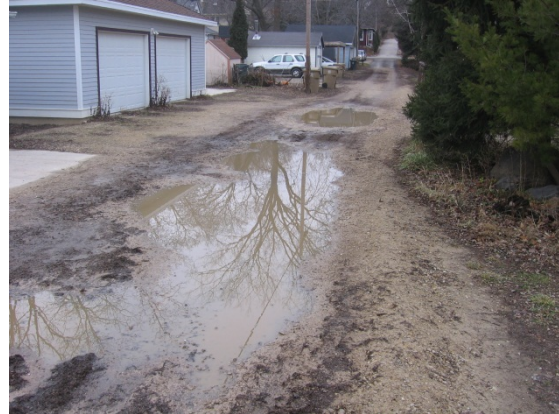
Water pooling issues in Section G Alley (poor condition)
