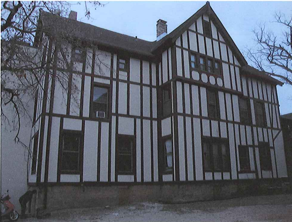
Image showing the east exterior of the building. The floor deformations are occurring generally in the longer joist spans of the middle third of the building; in the section under the east west framed gable.
