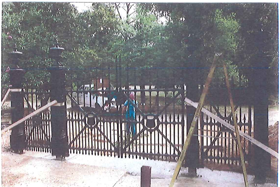
1999 Restoration of historic gates by Robinson Iron Corp, Alexander City, AL, www.robinsoniron.com
