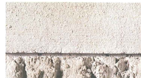
Smooth banding areas in the precast panels.
