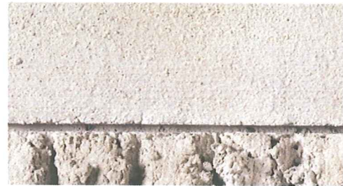
Smooth banding areas in the precast panels.
