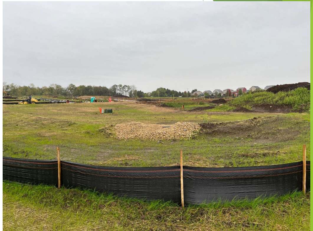
Acacia Ridge Erosion Control
