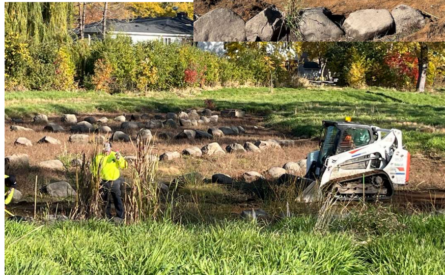
Nautilus Sand Filter Rejuvenation
