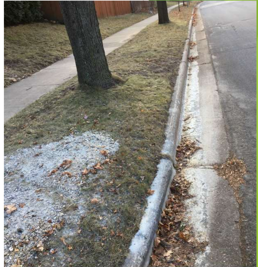
Concrete washout in curb
