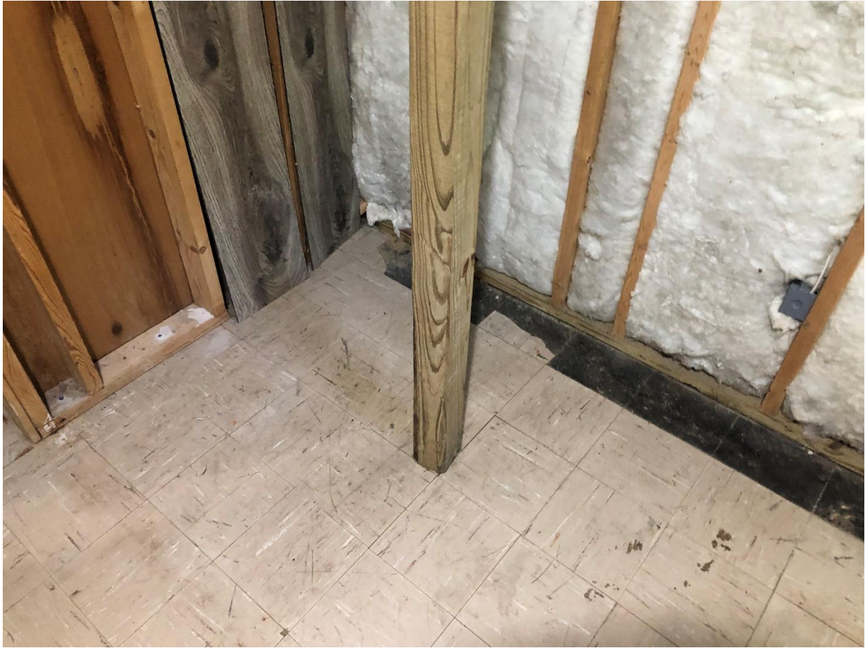
Image showing lack of attachment and lack of foundation at the base of wood columns.
