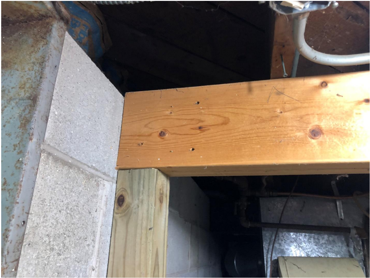
Image showing lack of appropriate structural attachment from the beam to the column. In addition, fastening should also be present at the joist framing to the wood beam.
