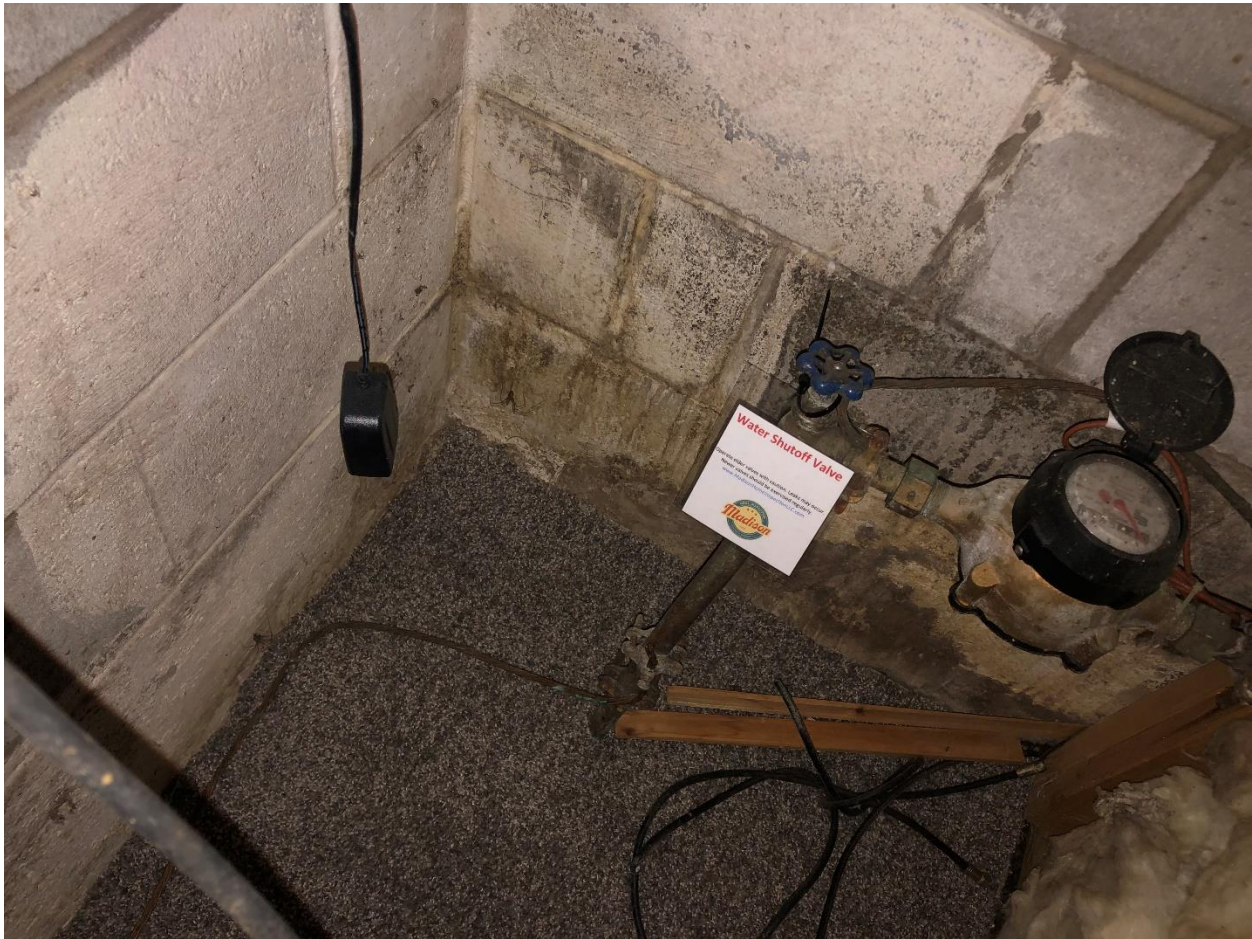
Image showing water staining on the base of the exterior foundation wall
