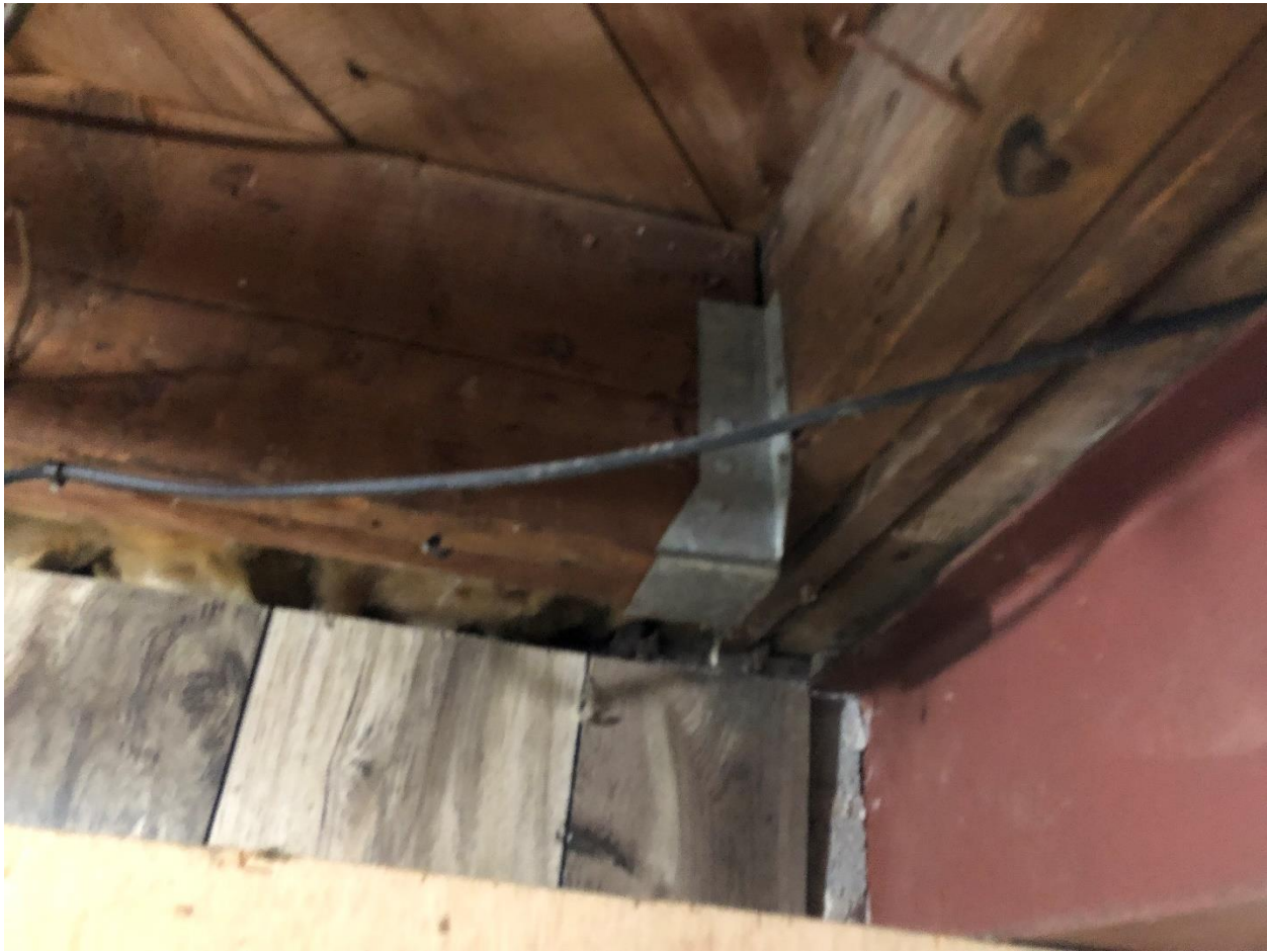
Inappropriate connection at hanger to supporting member.
