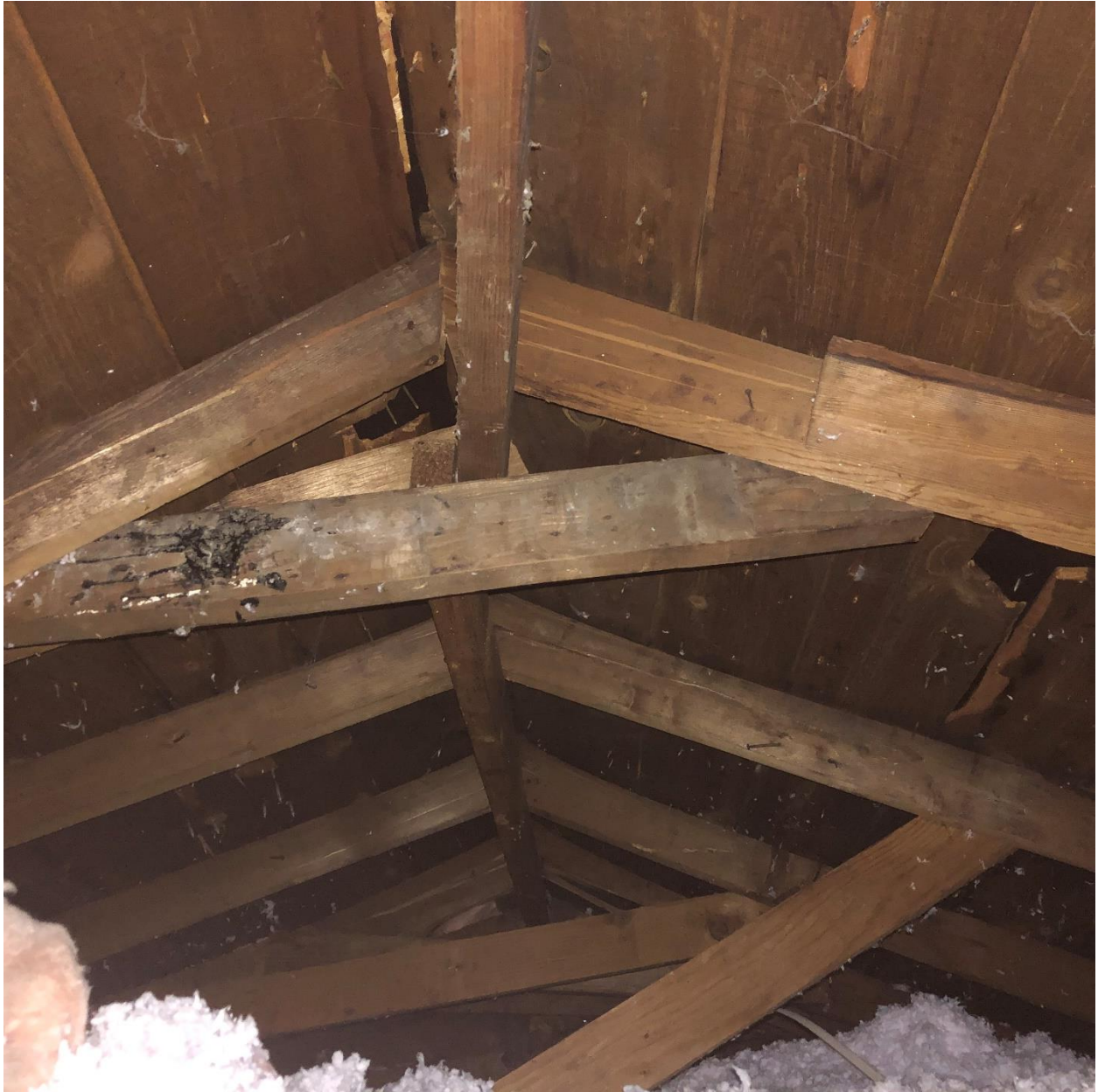
Image showing cracked rafters and cobbled roof framing
