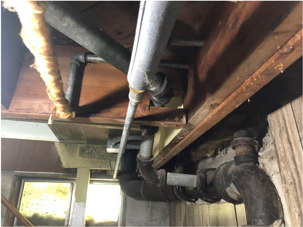
Image showing significant cut out notch at floor header/joist.
