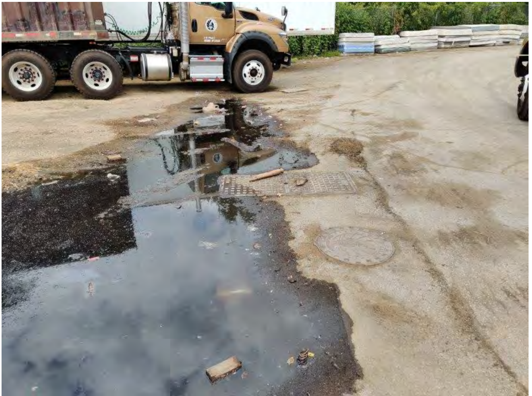
S-2 Storm Inlet
