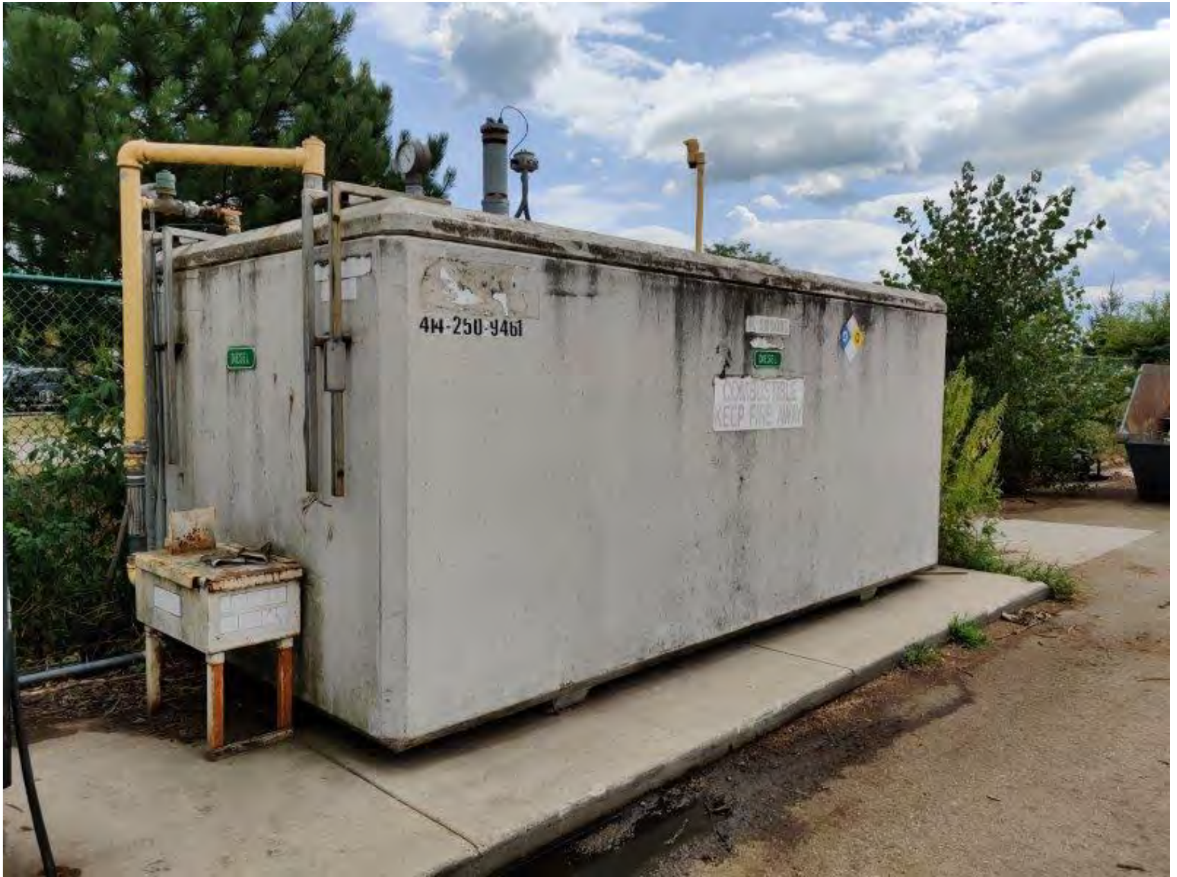
M-4 Fuel Storage and Fuel Pump
