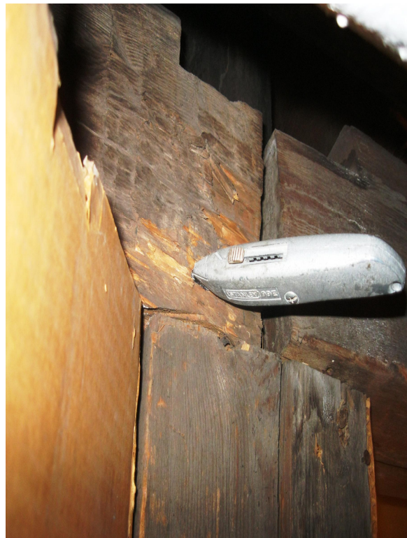
Photo 2 – Poor fit up and wood density at 1 st floor beams and column
