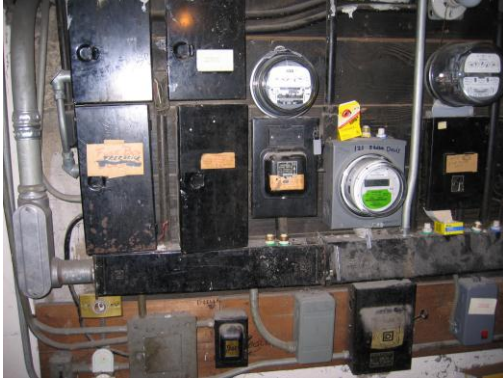
A portion of the older electrical service equipment in the Basement.
