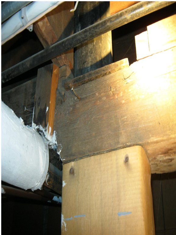
Photo 1 – Notched 1 st floor beam requiring replacement
