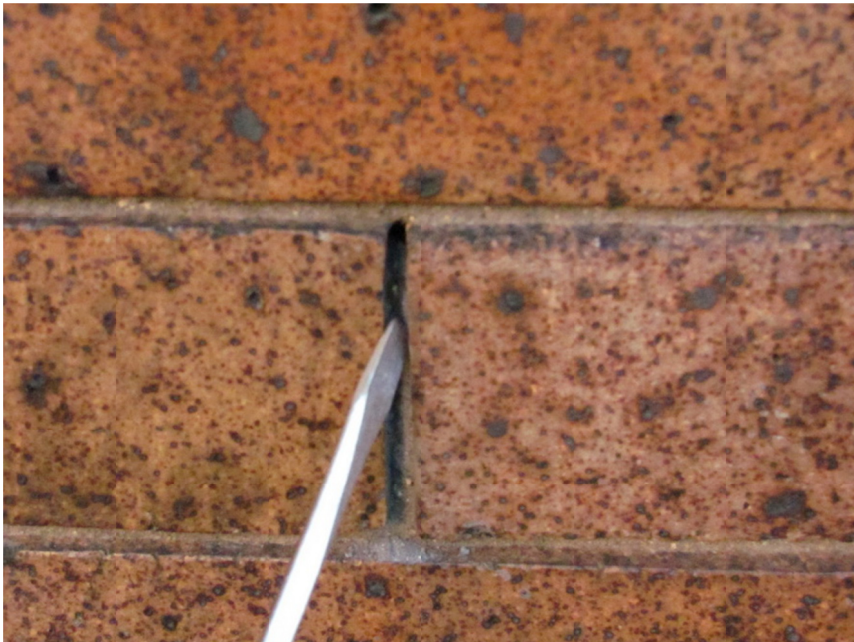
Figure 4. Occasional open mortar joints were observed.
