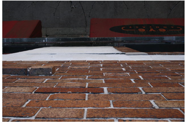
Exterior: View from roof of plaster-coated wall surface showing delamination of the plaster coating
