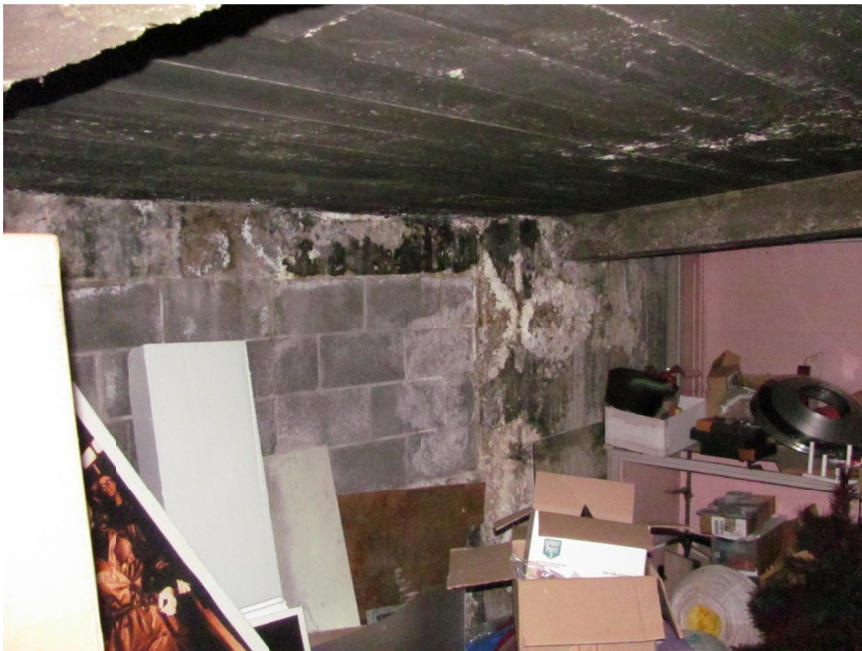
Figure 22. Efflorescence and water staining at the basement level below the entrance storefront.
