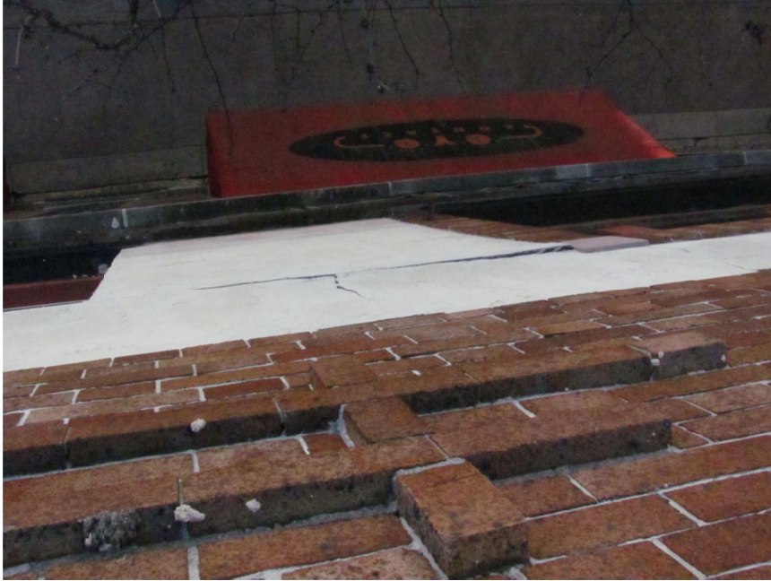
Figure 5. View from the roof of one especially large delaminated area of stucco observed near the middle of the facade.
