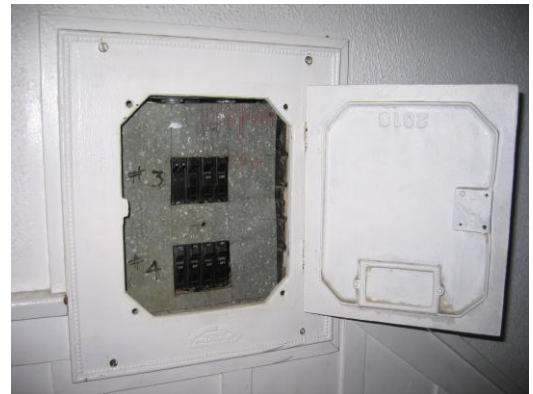
Third floor fuse panel converted to circuit breakers.
