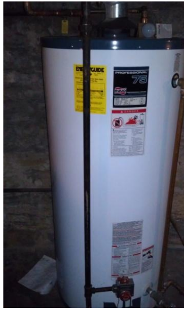
New water heater
