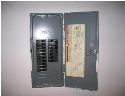
Electrical panel on 1 st floor retail.
