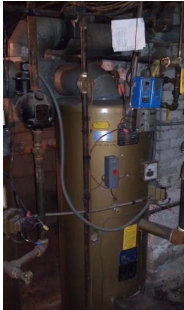
Hot water boiler
