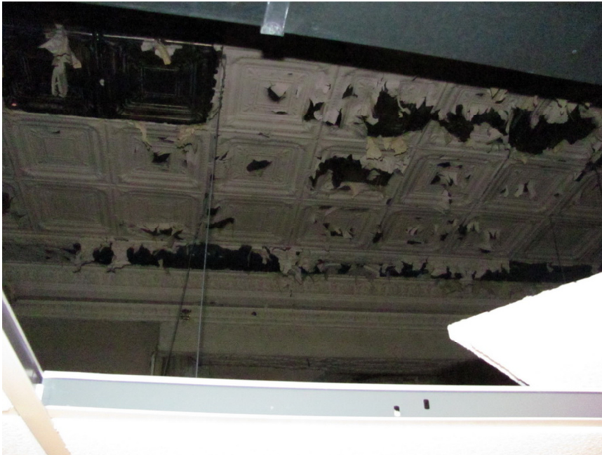
Figure 18. A suspended acoustic tile ceiling conceals other similar original pressed metal ceilings. The full extent of the pressed metal ceiling finish is not known.
