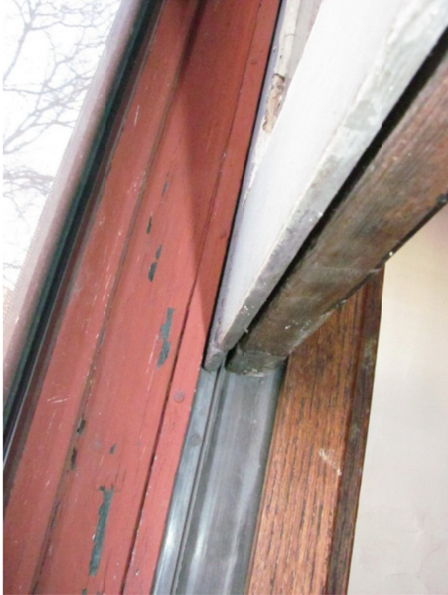
Figure 9. The original wood windows appeared intact and have been routed to receive galvanized metal weatherstripping.
