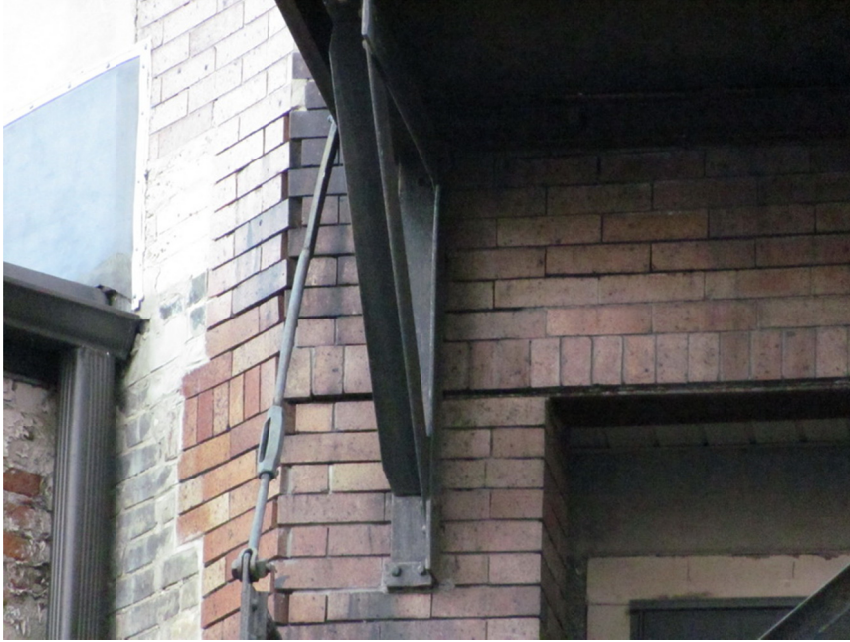
Figure 13. Surface corrosion and minor displacement of masonry associated with the bearing points of the lintels was observed.
