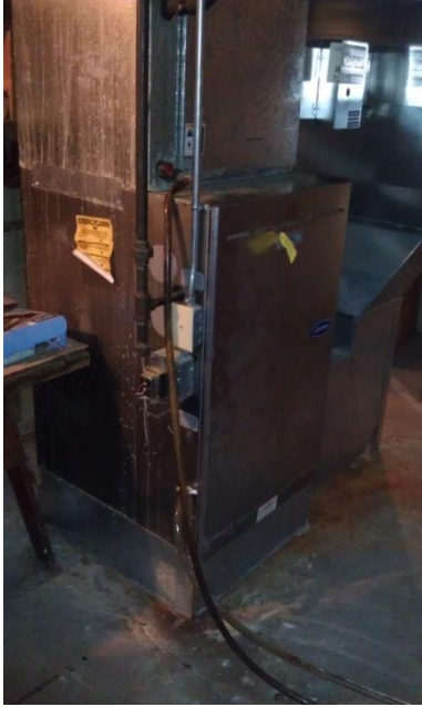
First floor furnace
