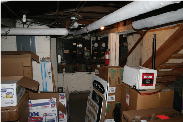
Basement: View of electrical
