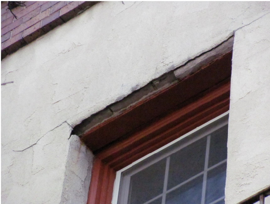
Figure 6. A portion of stucco has previously spalled at the head of the center third floor window.
