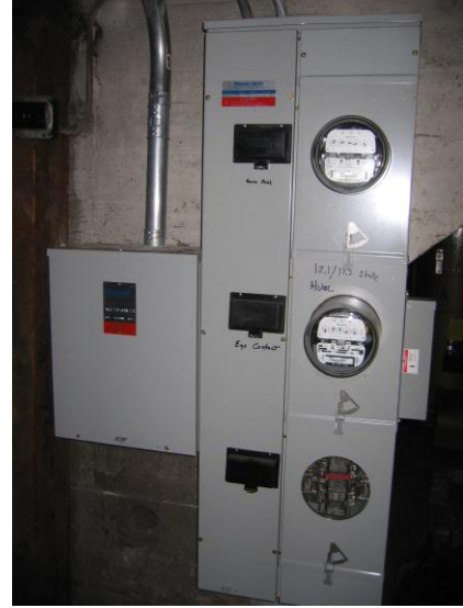
The newer electrical meters in the Basement.
