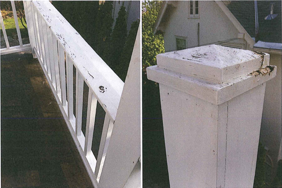
Photos 4 + 5: Existing painted wood railing. Proposed railing to match material, paint color, and detailing. Adjustments to vertical wood rail spacing to meet building code will be required.
