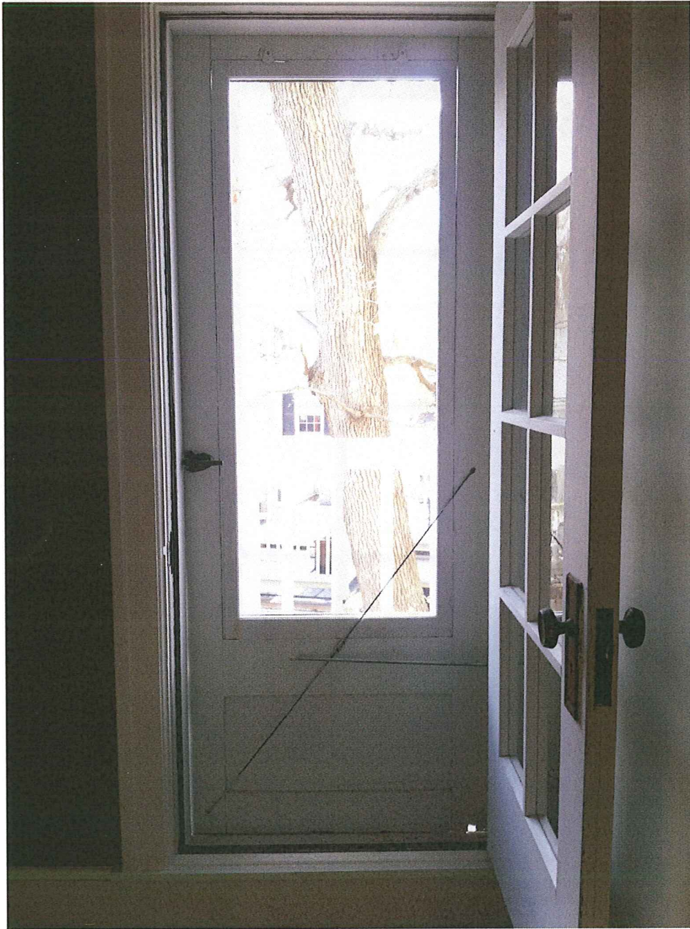
Photo 2: Existing painted wood door screen door to exterior porch at stair landing. Proposed screen door to match style, material, and paint color.
