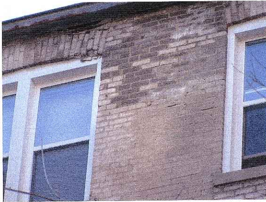
Water Damaged Bricks 433 Gilman Street March 10, 2006
