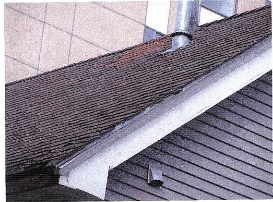
Rotten Shingles, Patched Roof 535 Conklin Place March 11, 2006
