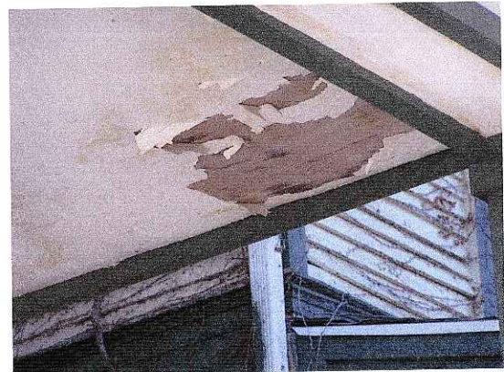
Rotted Ceiling 444 W. Johnson Street March 10, 2006
