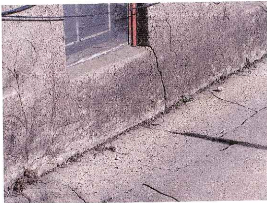
Cracked Foundation and Driveway 444 W. Johnson Street March 10, 2006
