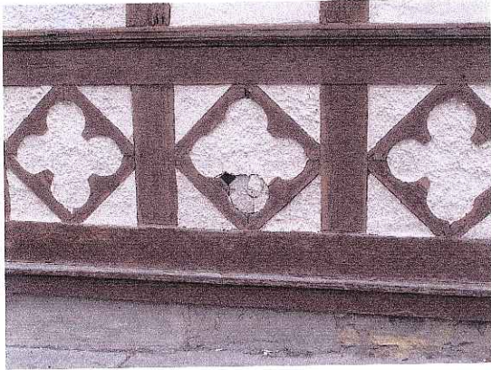
Rotted Trim, Broken Stucco 501 State Street March 12, 2006
