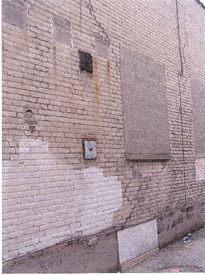
Wall Bolts, Wall Cracks, Boarded and Blocked Up Windows, Foundation Cracks 529 University Avenue March 11, 2006
