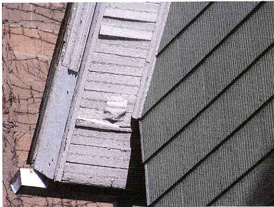
Rotten Soffit 414 W. Johnson Street March 10, 2006 March 10, 2006
