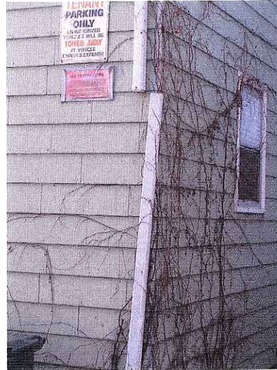
Broken Downspout 414 W. Johnson Street March 10, 2006
