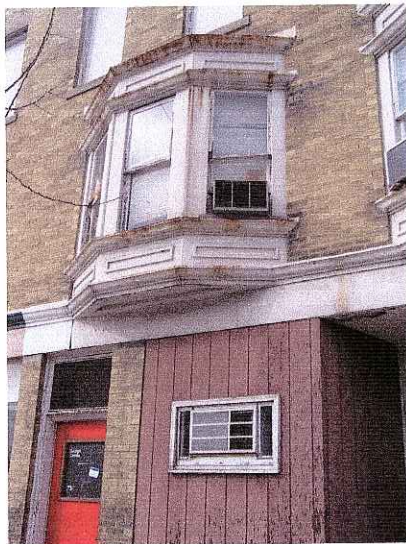
Cracked Wall, Bricked Up Windows, Deteriorated Window Frames 626 University Avenue March 14, 2006
