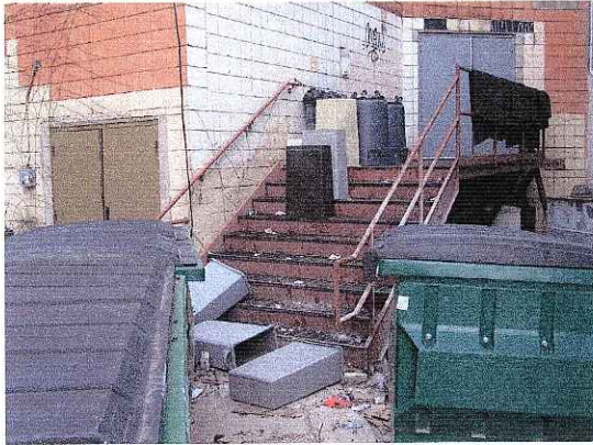
Exit Stairs Blocked 624 University Avenue March 14, 2006
