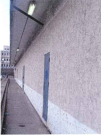
Missing Downspout, University Square March 11, 2006
