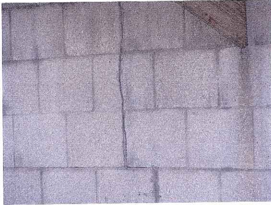
Cracked Foundations 304 Broom Street March 10, 2006
