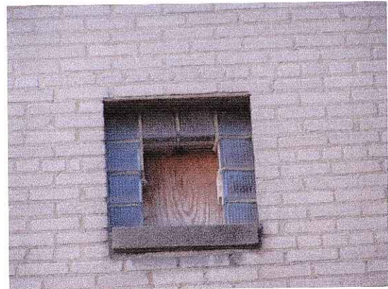
Broken Glass Block Boarded Up Window 433 Gilman Street March 10, 2006
