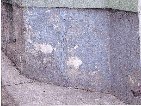
Cracked Foundation 414 W. Johnson Street March 10, 2006
