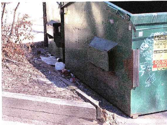
Unscreened Storage, Trash on the Ground Deteriorated Planter 454 Gilman Street March 14, 2006
