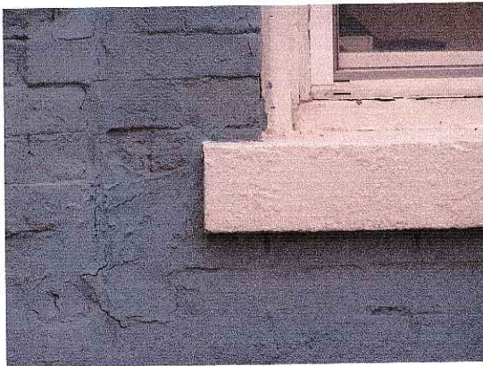
Deteriorated Brick Wall, Rotted Window Frame 450 W. Gilman Street March 12, 2006
