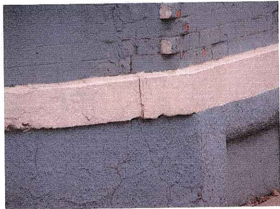
Cracked Foundation, Cracked Wall 450 W. Gilman Street March 12, 2006
