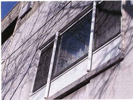
Window Frame Jacks 673 State Street March 14, 2006
