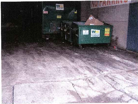
Broken Driveway University Square March 11, 2006
