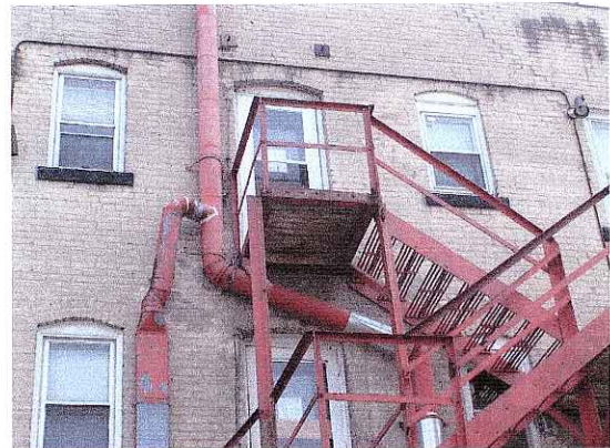
Wall Cracks, Wall Bolts, Deteriorated Porch Decks 614-612 University Avenue March 15, 2006
