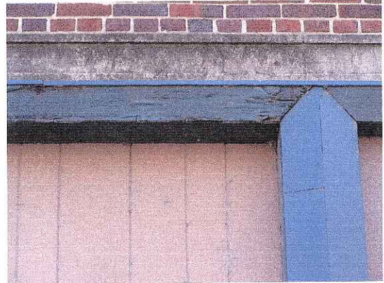
Store Front Rotted 645-651 State Street March 14, 2006
