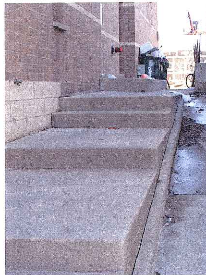
No Railing on Steps Trash on Ground in the Background 412 W. Johnson Street
