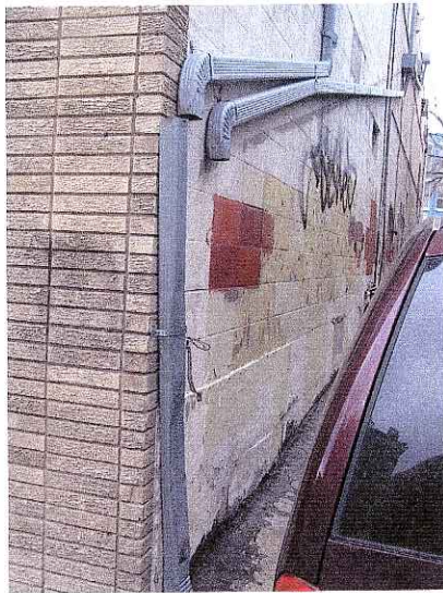
Downspouts Loose and Missing, Damaged Wall and Bulging Foundation 459 Gilman Street March 11, 2006
