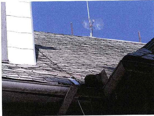
Broken and Loose Shingles 421 Gilman Street March 10, 2006
