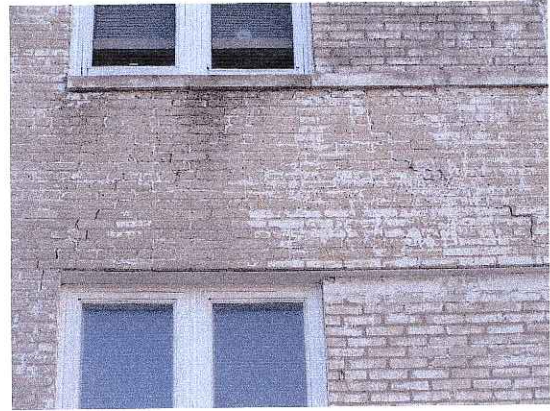
Cracked Wall 445 Gilman Street March 10, 2006
