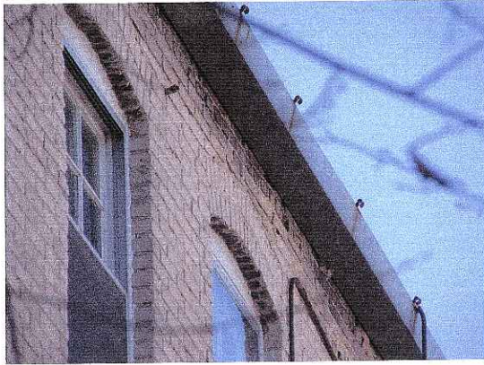
Deteriorated Bricks Under the Gutters 405 Lake Street March 14, 2006
