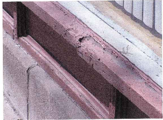
Deteriorated Window Frame 405 Lake Street March 14, 2006
