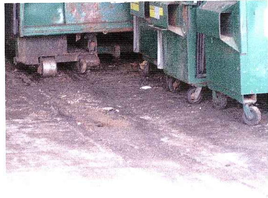
Grease Encrusted Floor University Square March 11, 2006
