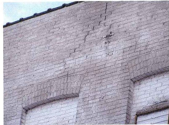
Wall Bolts, Broken Block, Cracked Wall, Windows Blocked 624 University Avenue March 14, 2006
