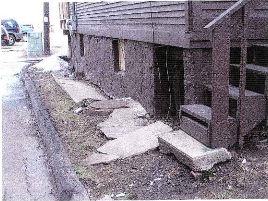
Dangerous Step, Deteriorated Siding, Boarded Basement Window, Parged Foundation, Destroyed Sidewalk 549 Conklin Place March 11, 2006
