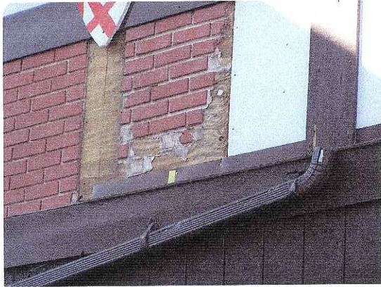
Missing Downspout, Missing Siding 603 State Street March 14, 2006
