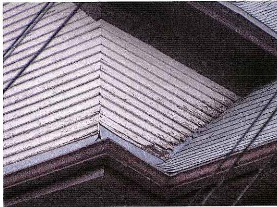
Rotted Clap Board 308 Bassett Street March 11, 2006
