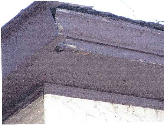
Deteriorated Fascia and Soffit 318 Broom Street March 10, 2006
