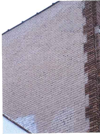
Cracks in the Wall 414 Francis Street, 511 State Street March 12, 2006
