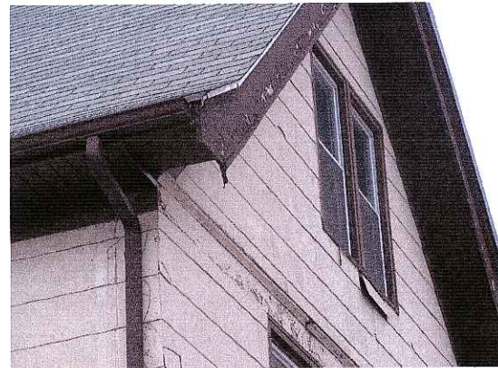
Rotted Fascia, Loose Siding 308 Bassett Street March 11, 2006
