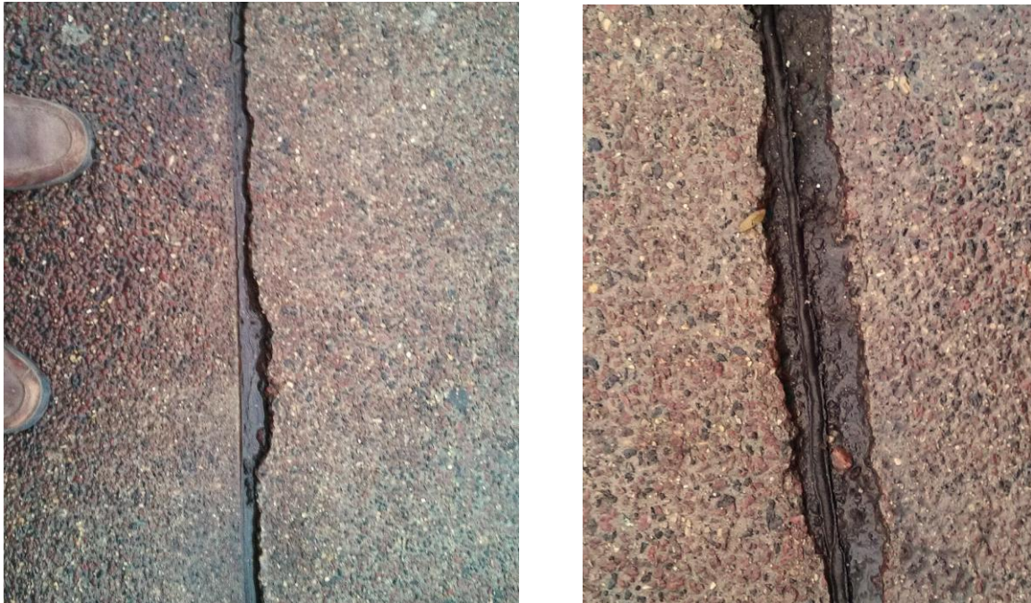
Figure 3. Cracking, spalling and raveling along joints
