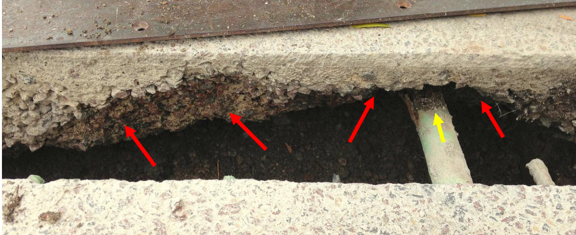
Figure 2. Oblique view of the slab showing deterioration of the slab bottom (red arrows) and corrosion of a dowel bar (yellow arrow).
