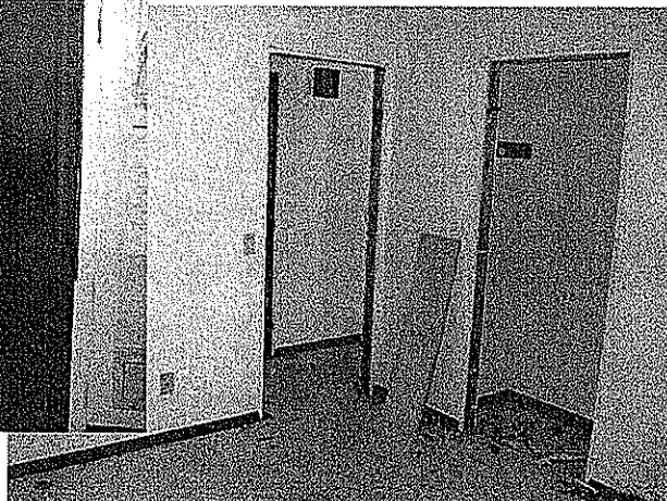
Doors and doorframes are missing. Bedrooms in fair condition.
