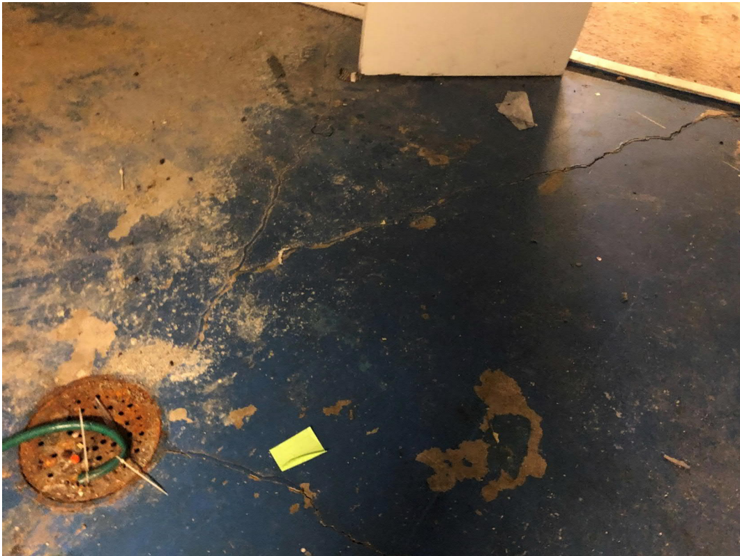
Basement - note floor crack
