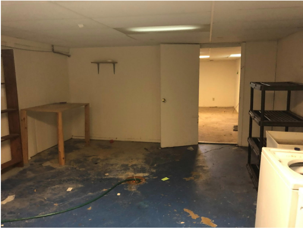
Basement - note floor crack
