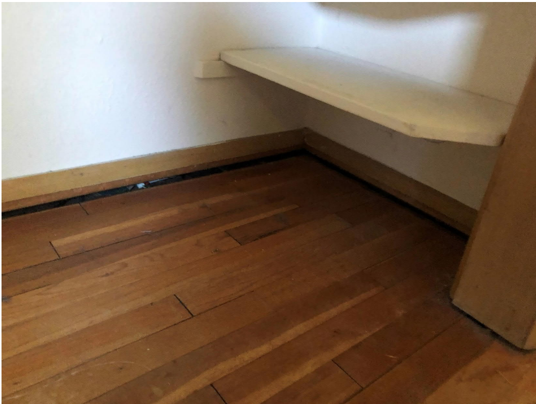
Bedroom closet - Floor settlement gap between floor and baseboard
