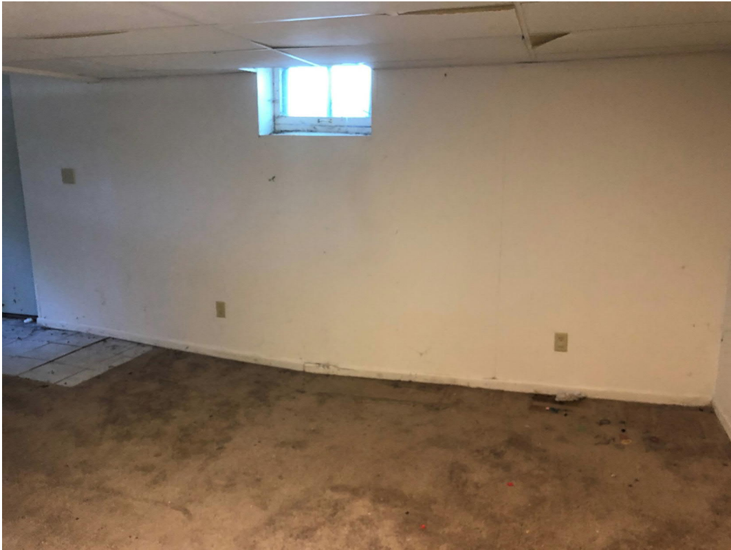
Basement - note floor slope along wall, carpet covering floor.
