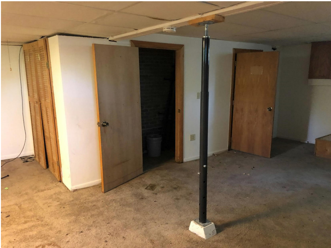
Supplemental floor support added - note separation of wall from ceiling. Door frames are racked and doors swing open.
