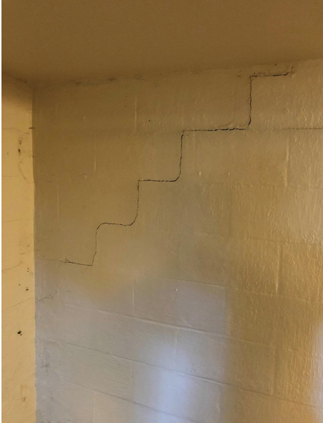
Foundation wall crack
