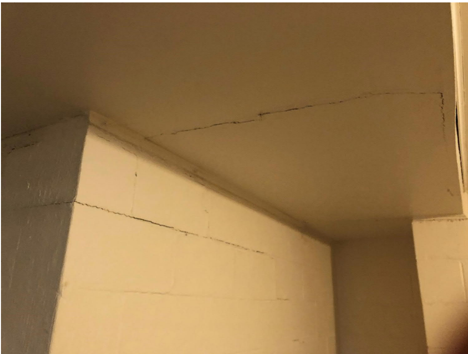
Foundation wall and ceiling cracks
