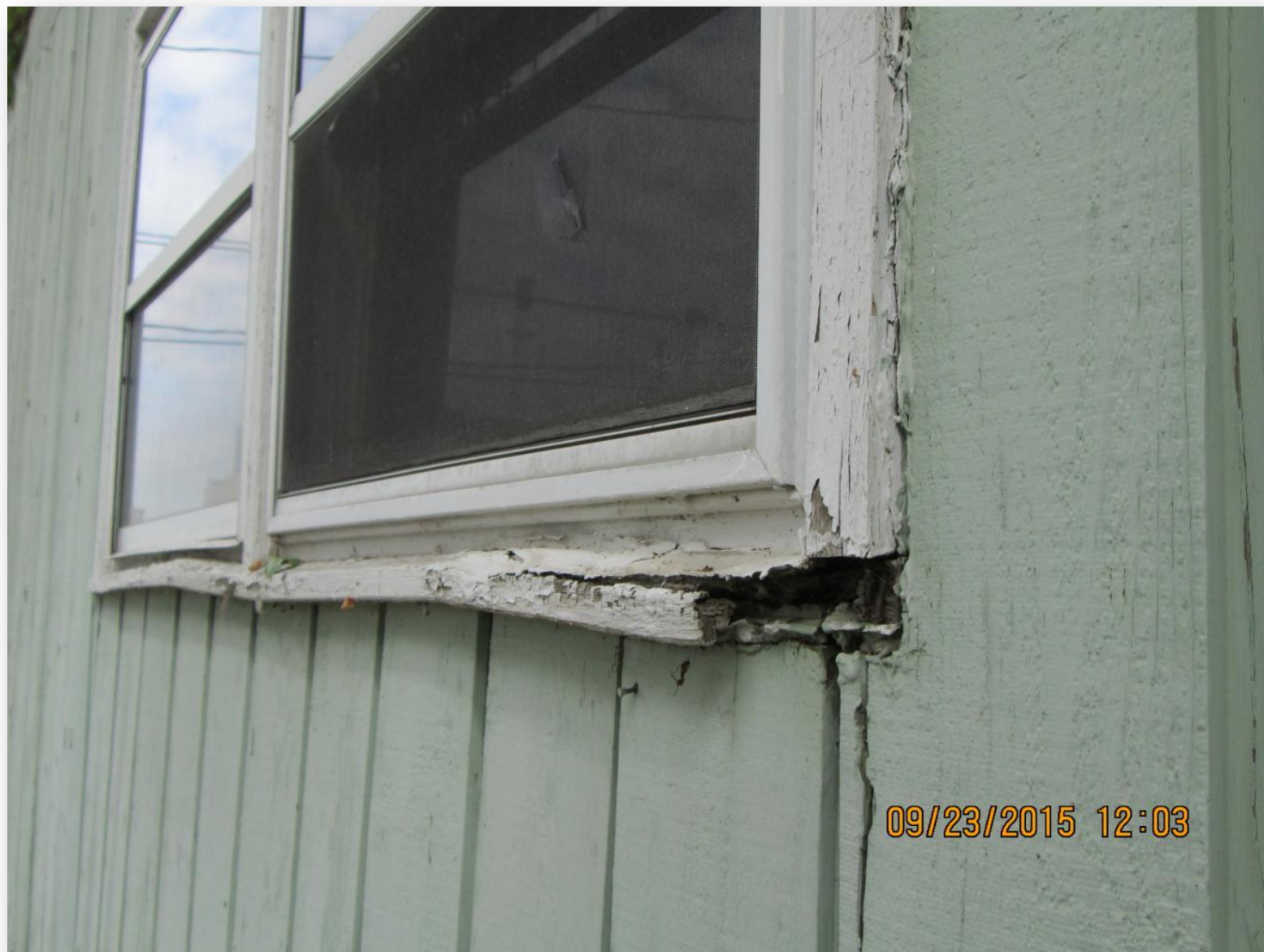
ROTTED WEST, FIRST FLOOR WINDOW SILLS (2)
