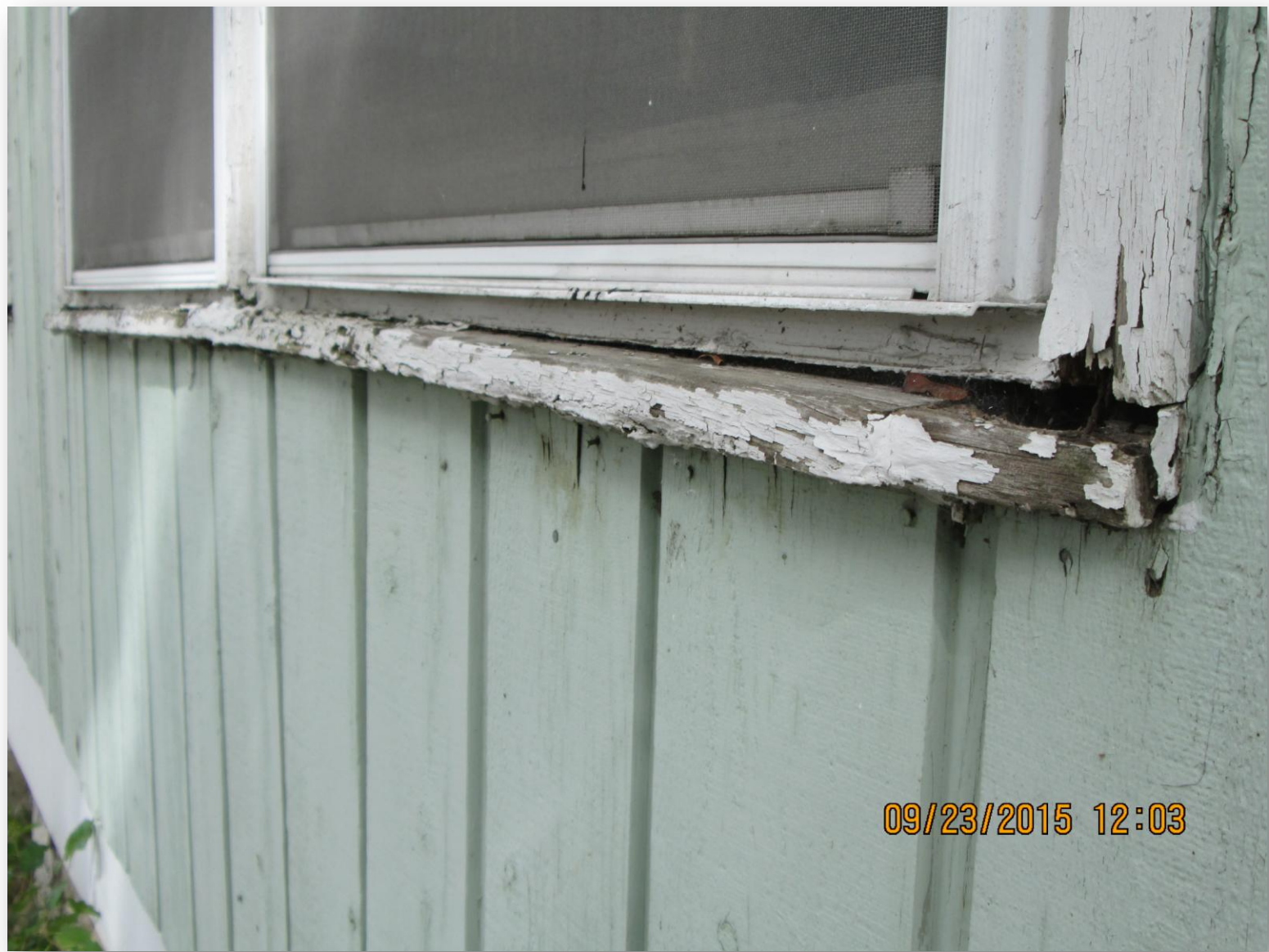
ROTTED WEST, FIRST FLOOR WINDOW SILLS
