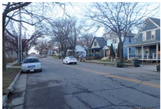
North Baldwin looking northwest (cracks, patching)
