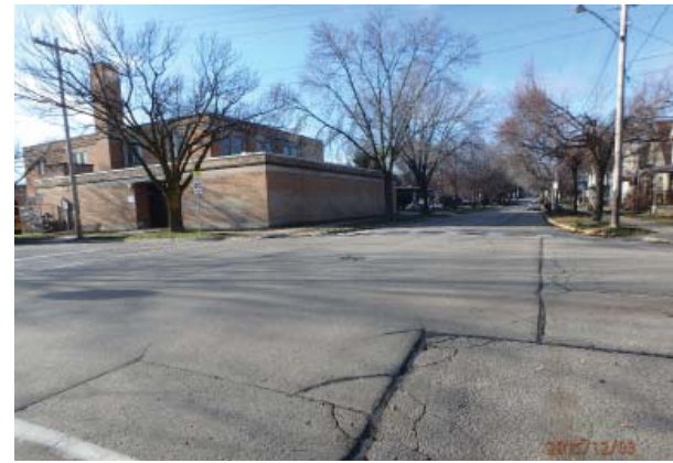
North Ingersoll at East Mifflin (cracking, patching)
