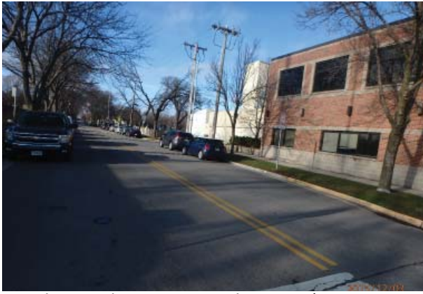
North Brearly at East Washington (paint chipping, pavement chipped)
