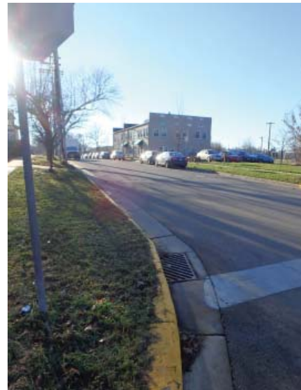
South First at East Main looking southwest (cracking, paint chipping)
