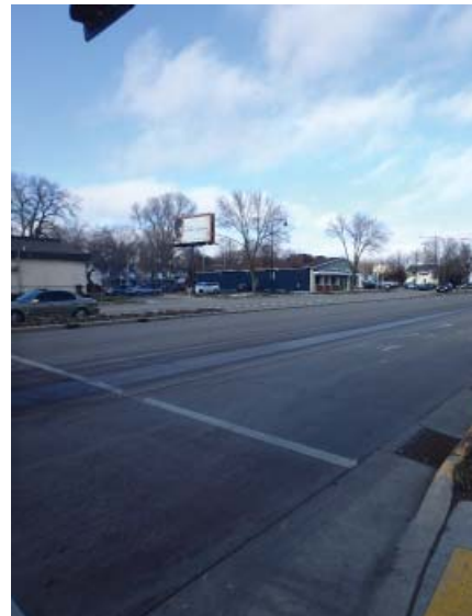
East Washington at South Ingersoll looking northeast (paint faded/worn away at crosswalk, chipping)
