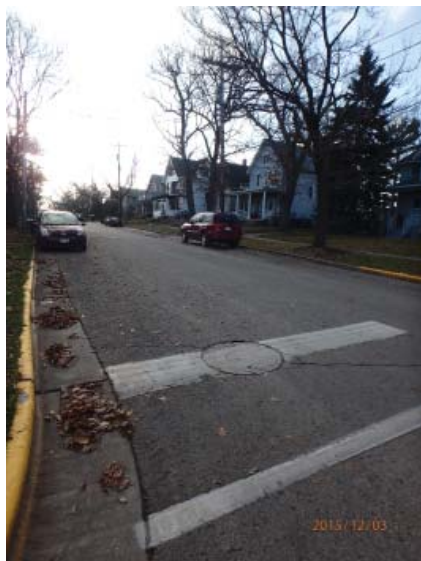
East Dayton looking southwest (cracking, paint chipped, discoloration)
