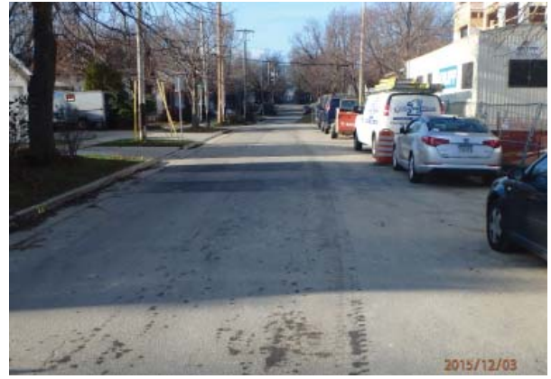
North Few at East Washington looking northwest (cracking, gravel pile on street)
