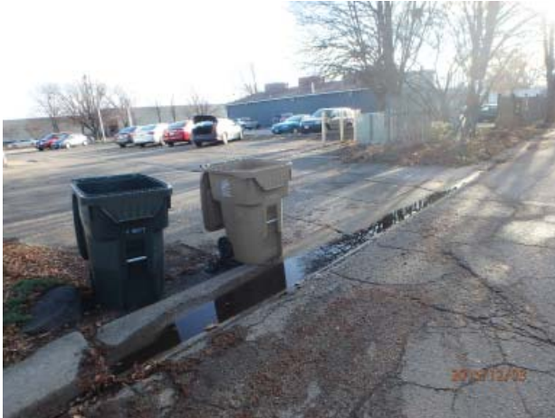
Curtis Court (water pooling in gutter, cracking)
