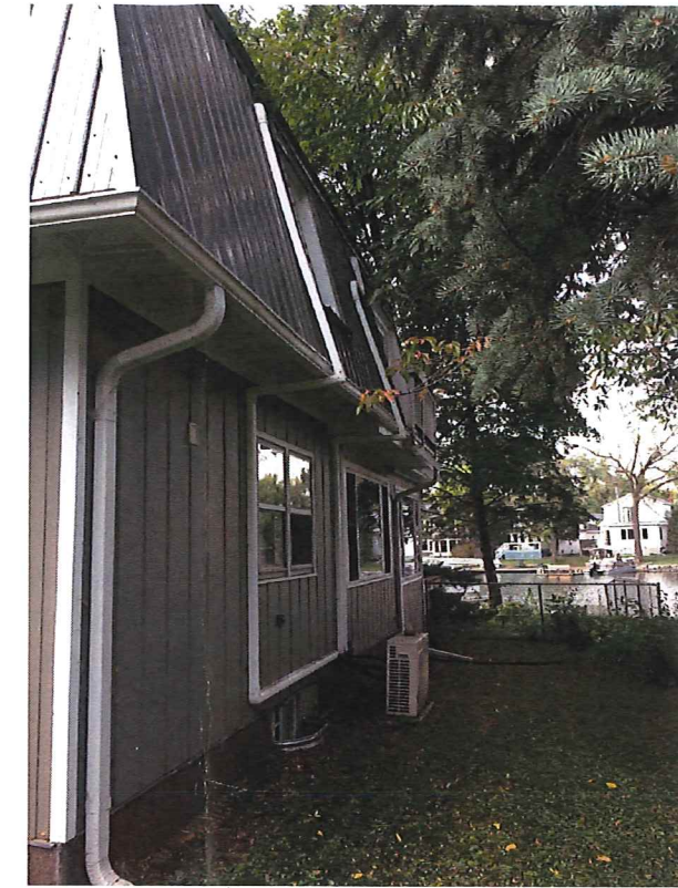
Photo of affected area on East side of house
