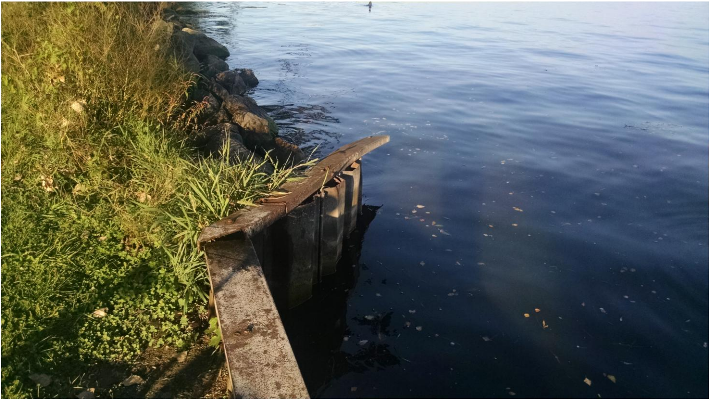
Photograph 2: Photograph taken on September 9, 2014, shows the general condition of the bulkheads. Although the metal is still sound, the caps have been displaced, exposing sharp metal edges. It is unknown when the bulkheads were installed, or what their original purpose was.
