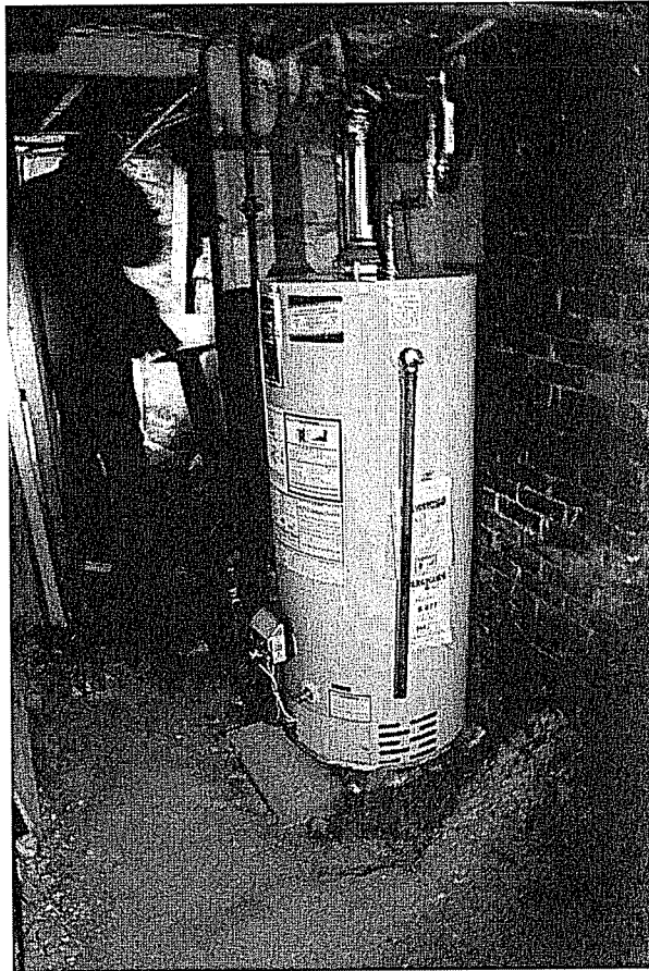
2. Basement – Water Heater
