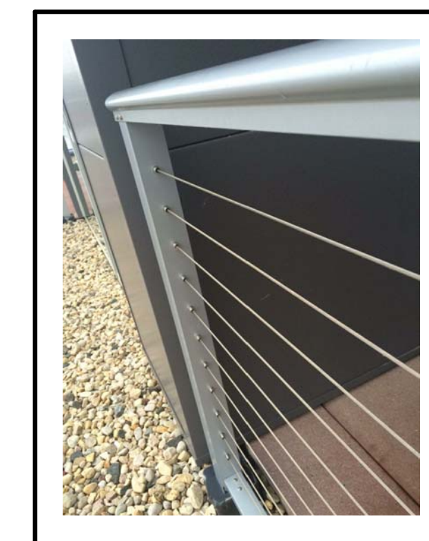
ALUMINUM & STAINLESS STEEL RAILING: NATURAL ANODIZED AT LIVE/WORK & DARK BRONZE AND CONDOS
