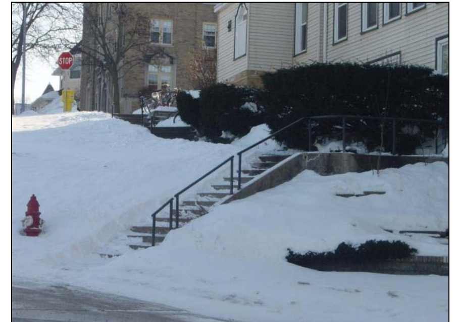
City Maintained Access is Not ADA or Code Compliant
