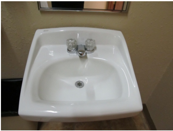
Sink handles are not ADA compliant. Improvements will replace handles with paddle type faucets.
