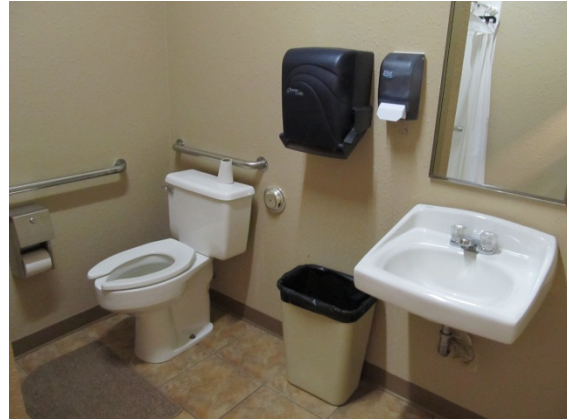
Paper towel dispensers and soap dispensers should be lowered
