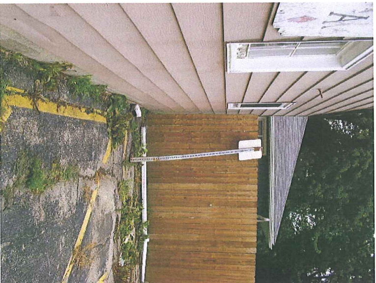
Accessible parking stall not permanently installed, facing backward against fence.
