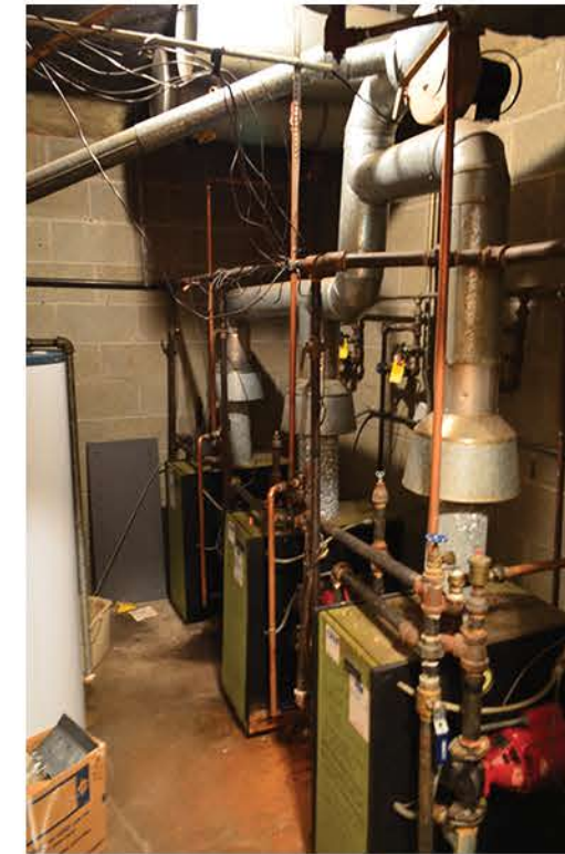
Mechanical room within original building
