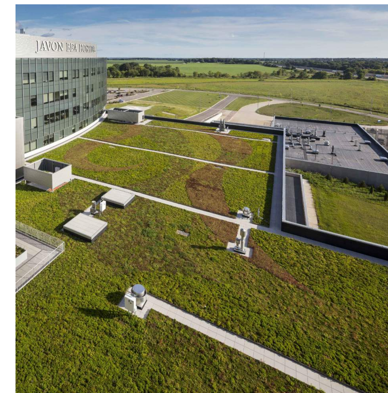
Typical rooftop / penthouse green roof with 2' clear zone around outside edges and mechanical units. Includes additional paver walkways for maintenance access.
