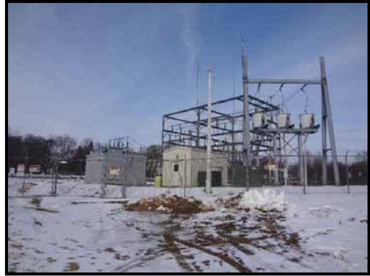
Electrical Substation (Directly Northwest of Site)
