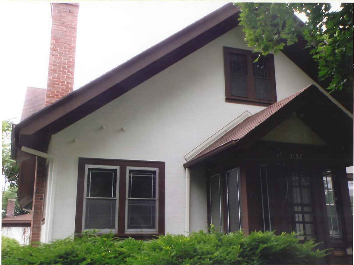
Second story front window to be replaced.
