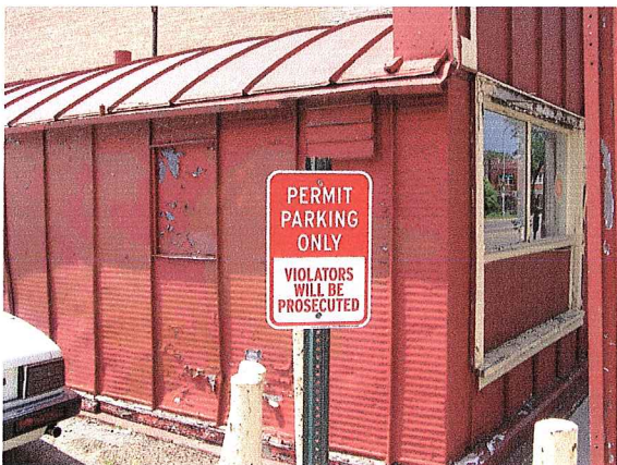
2033 Atwood Avenue Obsolete Building June 2, 2005
