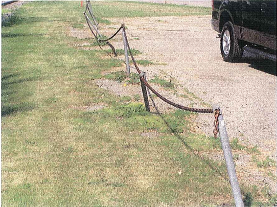
2240 Winnebago Street Broken Boundary Fence June 2, 2005
