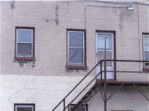
3820 Winnebago Street Cracked Wall June 2, 2005
