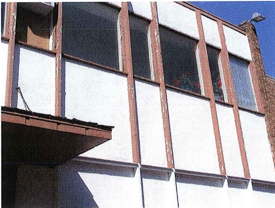
1915 Winnebago Street Deteriorated Window Frames May 30, 2005
