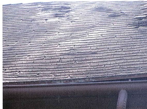
2146 Winnebago Street Deteriorated Shingles June 2, 2005
