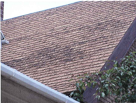
2146 Winnebago Street Deteriorated Shingles June 2, 2005
