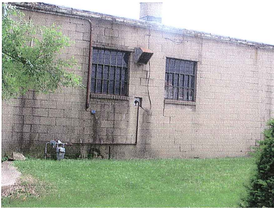
2652 East Washington Avenue Cracked Wall Water Damaged Wall June 6, 2005
