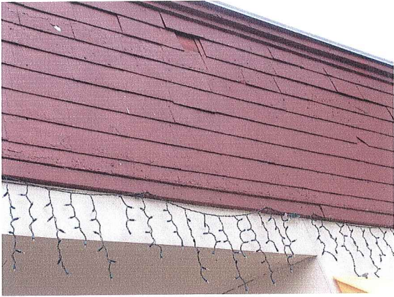
2422 Winnebago Street Deteriorated Siding Missing Siding June 3, 2005
