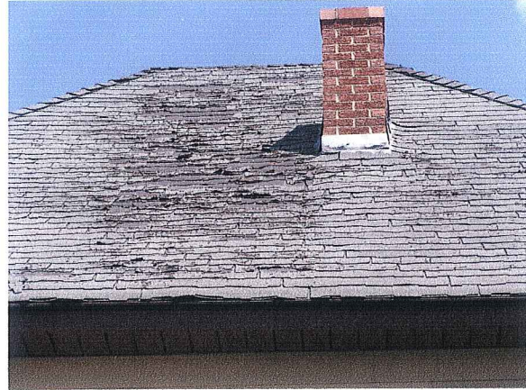
1833 Winnebago Street Deteriorated Shingles May 30, 2005
