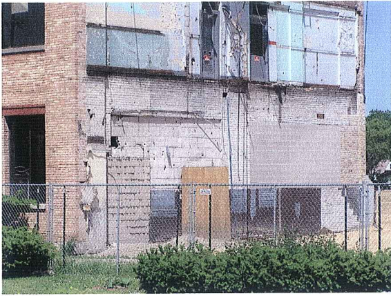
2317 Winnebago Street Hole In The Wall Second Story Door With No Porch Blocked-up Window June 6, 2005
