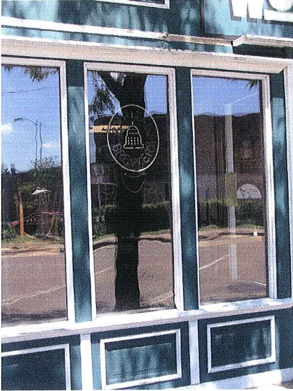
1980 Atwood Avenue Deteriorated Paneling Deteriorated Window Frame Trim Missing May 30, 2005
