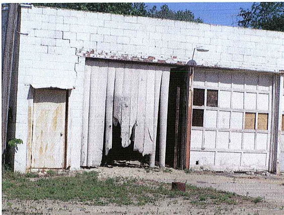
149 Waubesa Street Missing Door Windows Missing From Door June 6, 2005
