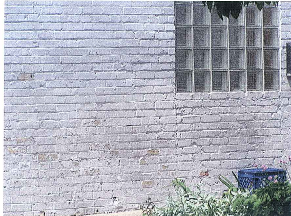
2007 Atwood Avenue Deteriorated Bricks Blocked-up Window June 2, 2005
