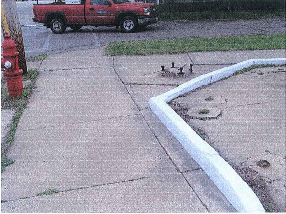
11 South Fifth Street Abandoned Sign Base Inside Walk Area With Exposed Electric Wires June 2, 2005
