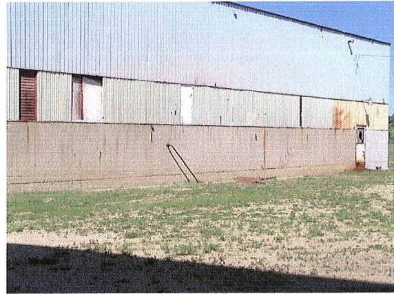
149 Waubesa Street Rusted Siding Siding Missing June 6, 2005
