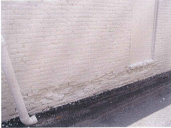
2017 Winnebago Street Deteriorated Brick Pieces of Brick on the Ground June 2, 2005
