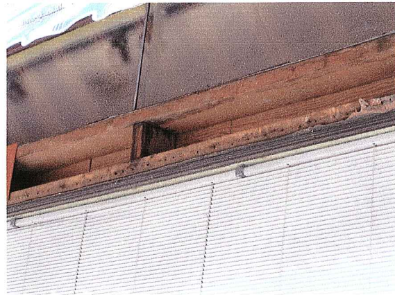
1947 Winnebago Street Panel Missing May 30, 2005
