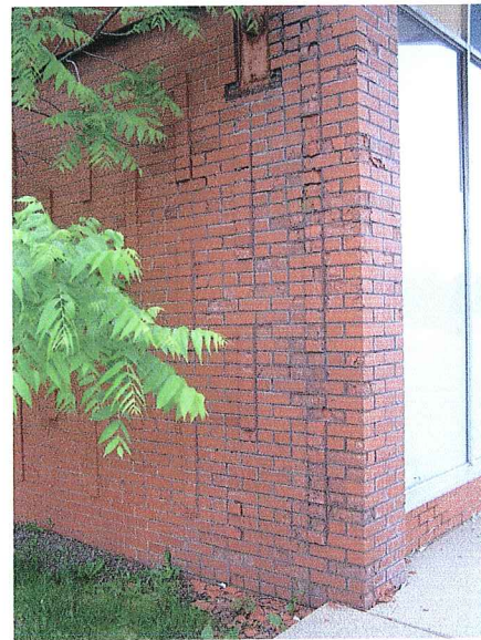
2525 East Washington Avenue Deteriorated Brick Pieces of Brick Lying on the Ground June 3, 2005
