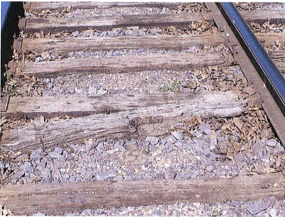
Between Corry and Winnebago Broken Ties June 6, 2005
