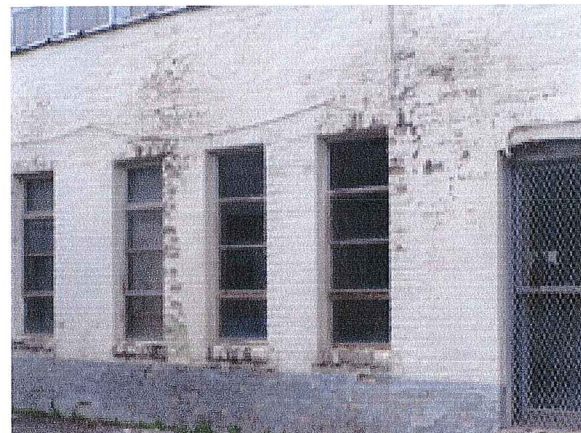
206 Waubesa Street Deteriorated brick May 4, 2006
