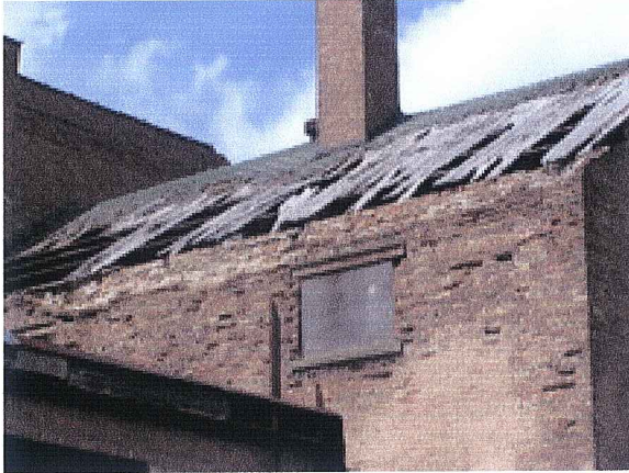
3244 Atwood Avenue Roof rotted away May 4, 2006
