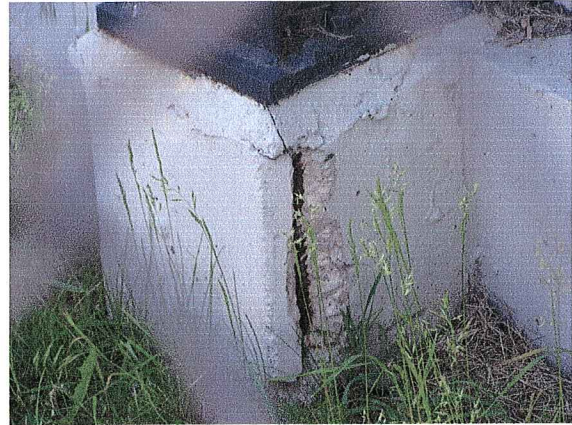
110 Waubesa Street Cracked Beam Support June 6, 2005
