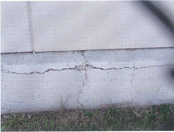
110 Waubesa Street Cracked Wall and Foundation June 6, 2005
