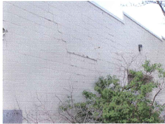
152 Dixon Street Cracked wall and blocked up window May 4, 2006
