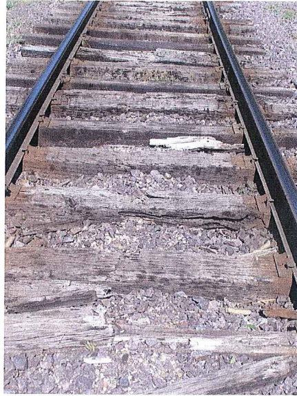
Between Corry and Winnebago Broken Tie June 6, 2005
