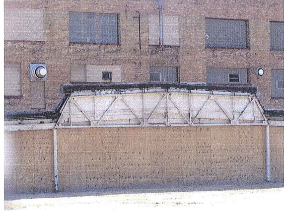
2317 Winnebago Street Wall Boarded Up Blocked-up Windows June 6, 2005
