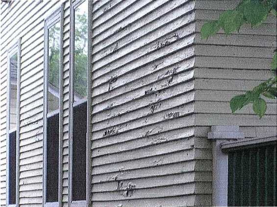
2303 East Washington Avenue Deteriorated Siding June 3, 2005
