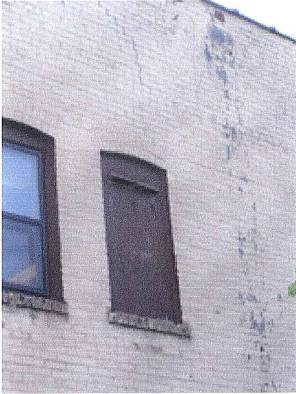
201 Waubesa Street Cracked wall, blocked up window May 4, 2006
