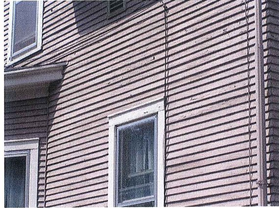
2142 Winnebago Street Deteriorated Siding Deteriorated Window Frame June 2, 2005
