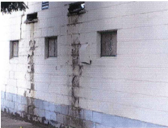
206 Waubesa Street Water damage and cracked wall May 4, 2006
