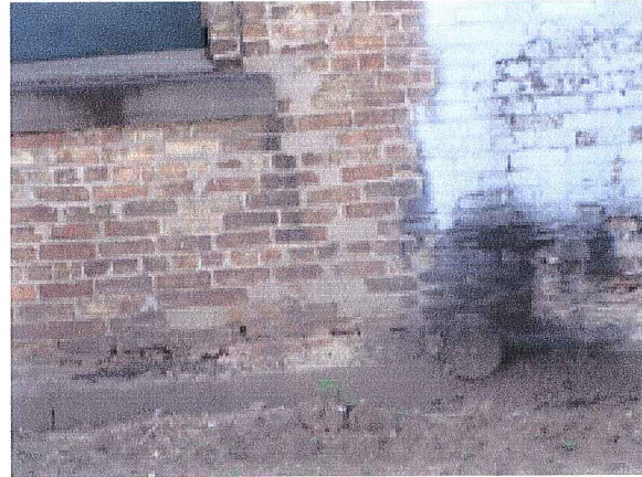
3244 Atwood Avenue Deteriorated all bricks, cracked wall May 4, 2006
