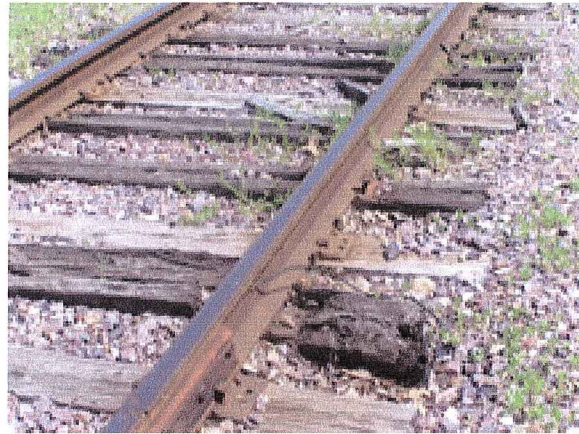
179 South Fair Oaks Avenue Rotten ties, broken ties, loose and missing spikes May 4, 2006
