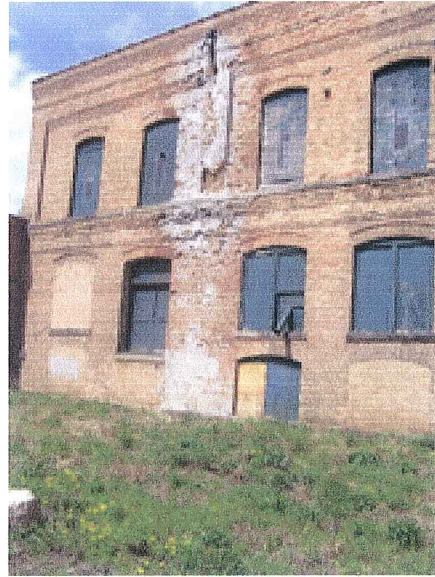
3244 Atwood Avenue Water damaged wall, boarded up windows, broken windows and deteriorated door May 4, 2006
