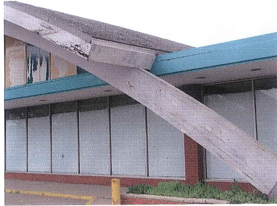
2525 East Washington Avenue Deteriorated Fascia Deteriorating Load-bearing Element June 3, 2005
