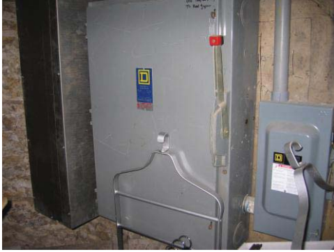
Building main disconnect.
