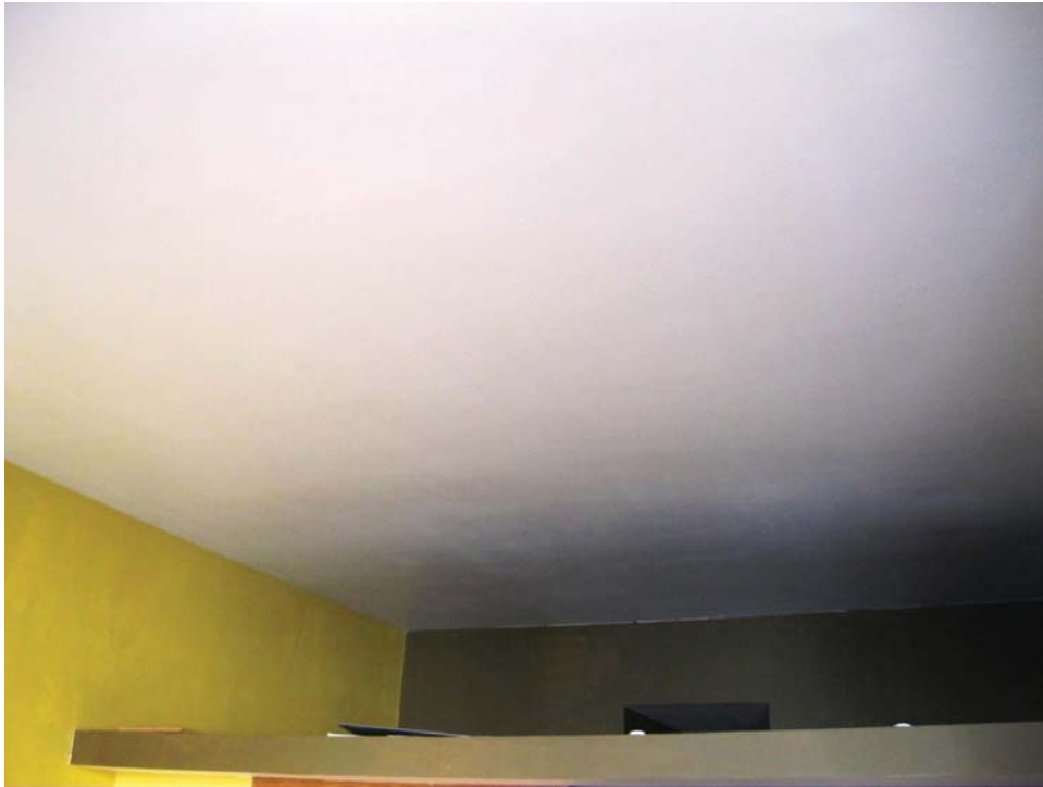
Photo 8 – 2 nd floor apartment ceiling
