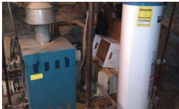
Hot water boiler and water heater
