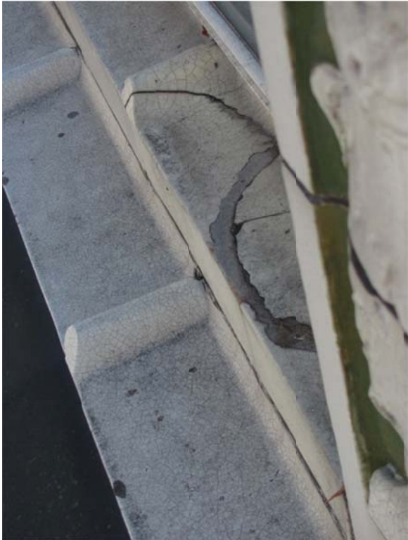
Figure 3. One cracked terra cotta window sill.
