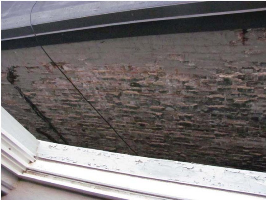
Figure 14. The masonry party wall as viewed from the adjacent building appeared to be in fair condition.
