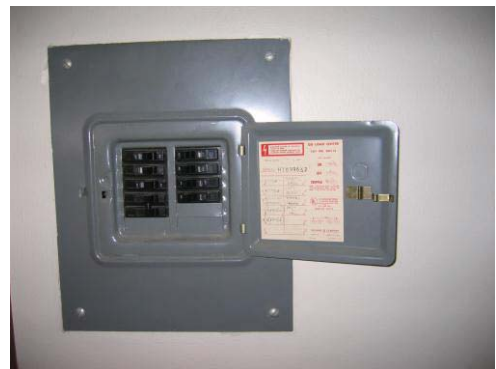
Electrical panel 125 1/2 State Street (2 nd floor apartment).
