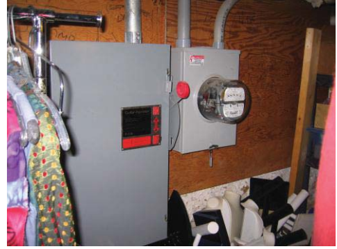
Basement electrical meter and disconnect.
