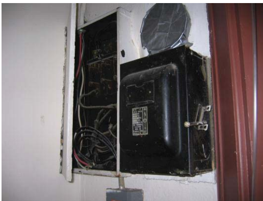
Knife switch and disconnect in 125 1/2 State Street (2 nd floor apartment).
