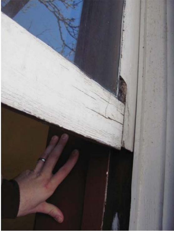
Figure 8. The wood windows are in fair condition, with some wood decay and displacement of window sash joinery.
