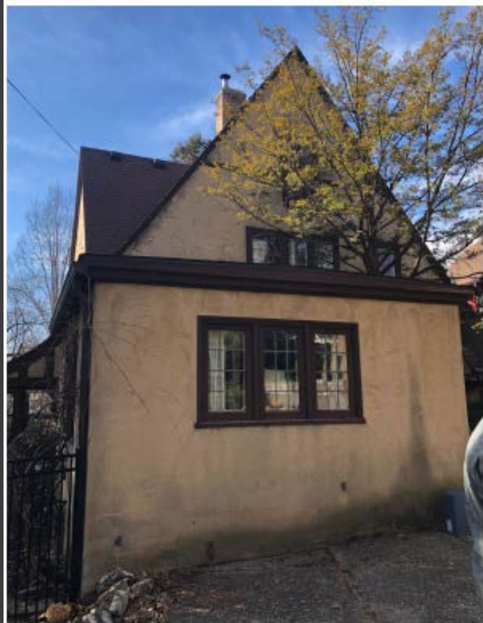
THIS PERSPECTIVE HINTS AT THE FORM OF THE SECOND LEVEL BATHROOM ADDITION ABOVE THE FLAT ROOF STRUCTURE
