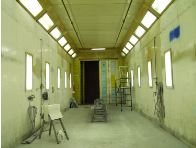
Figure 42: Low Overhead Clearance in Storage Area B
