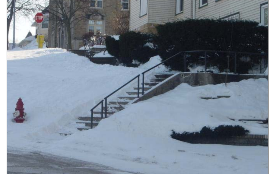
City Maintained Access is Not ADA or Code Compliant
