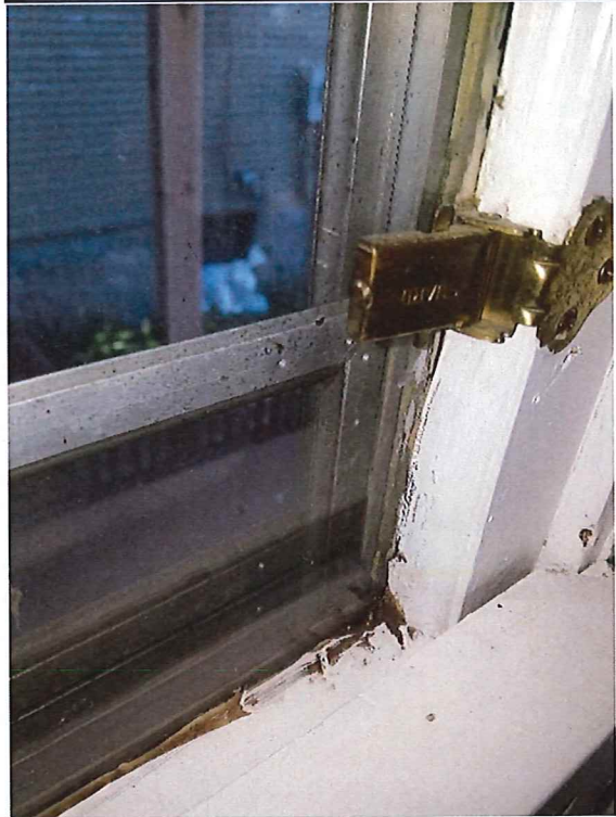
Window 1 1 st floor side near entry way Missing counter weight, alignment off, lower sash opens about 2 inches
