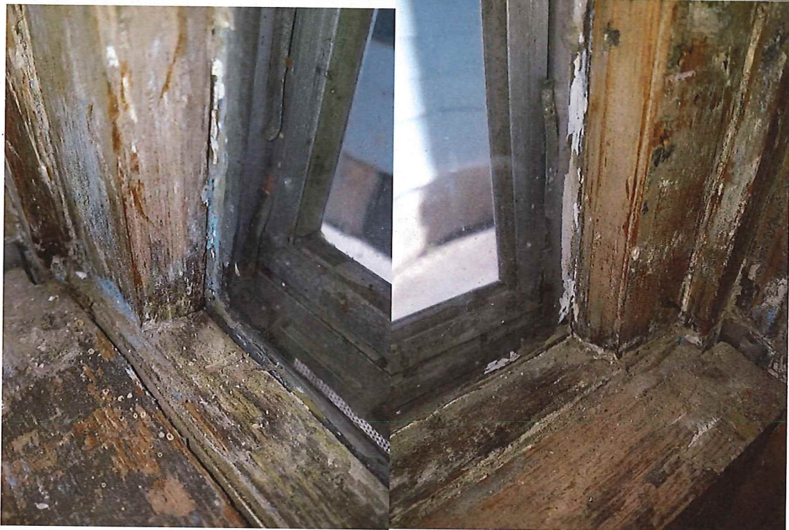
Window 10 1 st floor Kitchen Rot on all sashes. Missing storm window.
