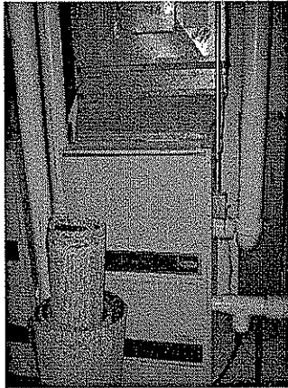
Forced Air Furnace Condition - Medium Quantity: 2
