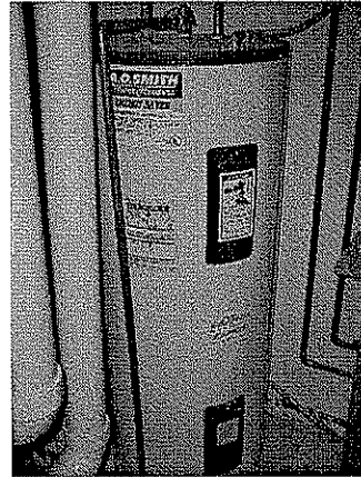
Water Heater Condition - Good Quantity: 1
