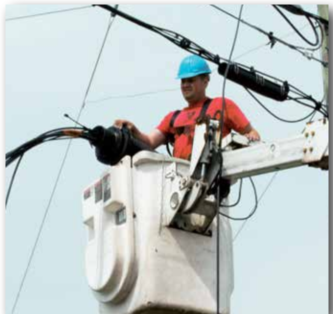
Danville, Va.'s use of its own utility poles for the nDanville network saved the city time and money.
