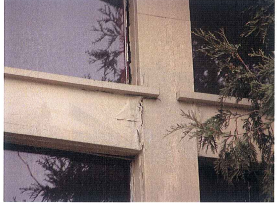
Deteriorated Frames, Loose Glazing March 30, 2006
