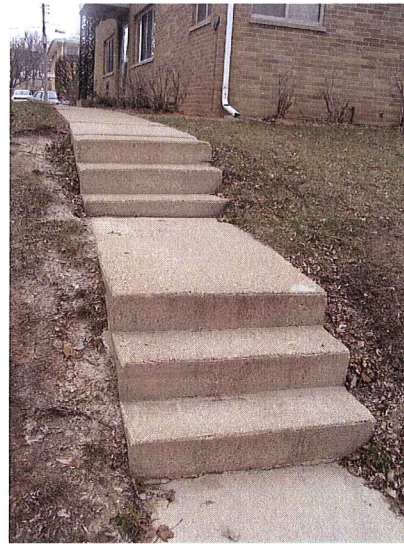
Steps Without Railing 2326-2322 Allied Dr March 30, 2006
