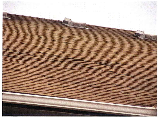
Deteriorated Shingles 2226 Allied Dr March 30, 2006
