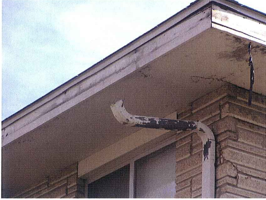
Downspout Off, Rotted Fascia, Soffet, No Gutter 2115 Allied Dr April 5, 2006
