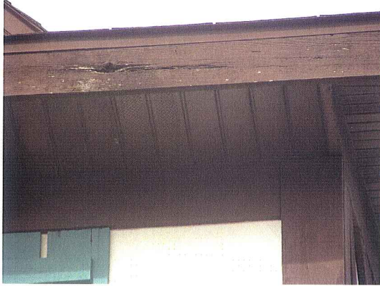
Rotted Fascia (Hole) 2211 Carling Dr April 13, 2006
