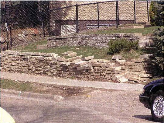
Deteriorated Retention Wall 4706 Genewein April 5, 2006
