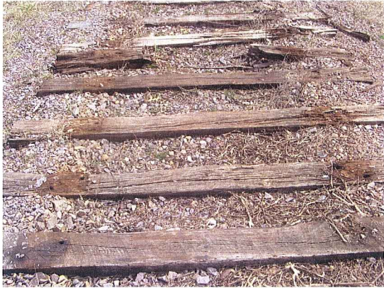
Rotten Ties, No Rails Railroad R-O-W April 11, 2006
