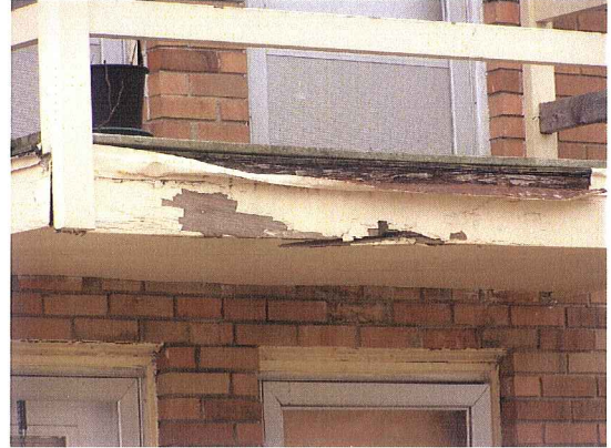
Rotted Porch Deck 2329 Carling Dr April 13, 2006
