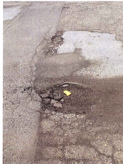
Pot Holes in Driveway 4649 Verona Rd March 30, 2006
