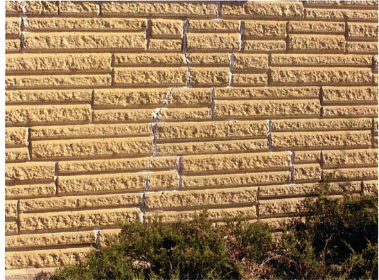
Wall Cracks 4709-4705 Genewein April 5, 2006
