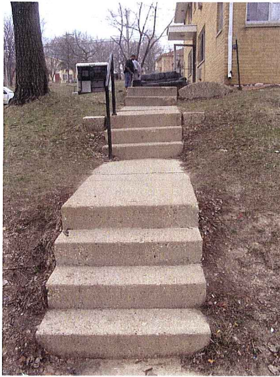
Steps Without Railing 2206 Rosenberry March 30, 2006
