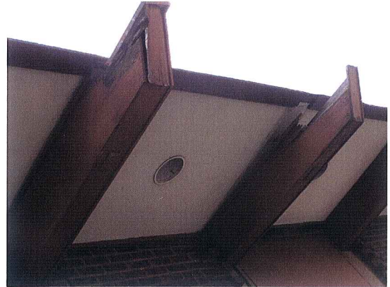
Rotted Fascia 4645 Verona Rd March 30, 2006
