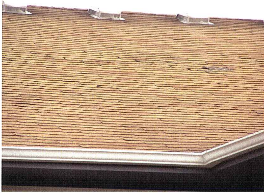
Deteriorated Shingles 2218 Allied Dr March 30, 2006
