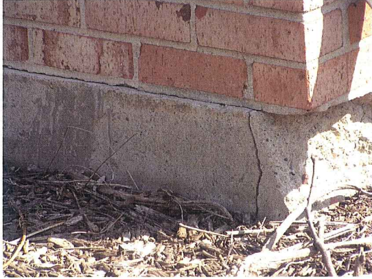
Foundation Broken and Cracked 2421-2417 Allied Dr April 10, 2006
