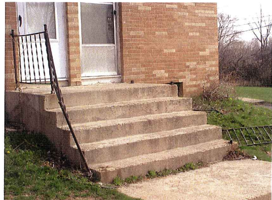
Railing Loose, Railing Missing (Lying on Ground) April 13, 2006
