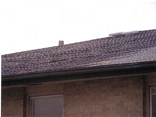
Deteriorated Shingles 2317-21 Carling Dr April 13, 2006
