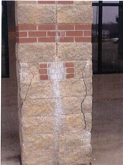
Cracks in the Pillar, Water Damage 4611 Verona Rd March 30, 2006
