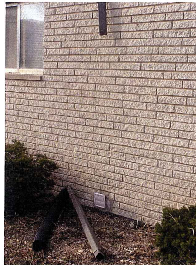
Downspout Off 2358-2354 Allied Dr March 30, 2006
