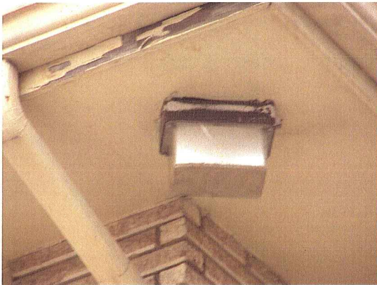
Deteriorated Porch Roof 2314-2318 Allied Dr March 30, 2006
