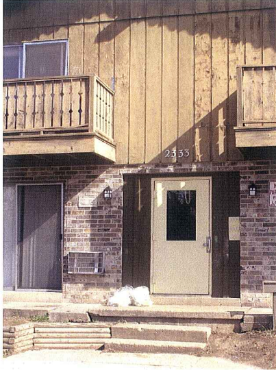
Lack of Railing on Steps, Rotted Wood Porch, Deteriorated Wood Walls 2399-2333 Allied Dr April 5, 2006
