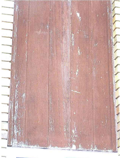
Deteriorated Wood Paneling 2118-2122 Allied Dr March 30, 2006
