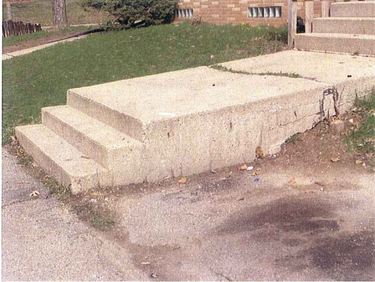
No Railings, Cracked Deck 2317-21 Carling Dr April 13, 2006
