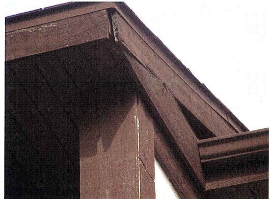
Deteriorated Fascia, Deteriorated Wood Frame 2201 Carling Dr April 13, 2006
