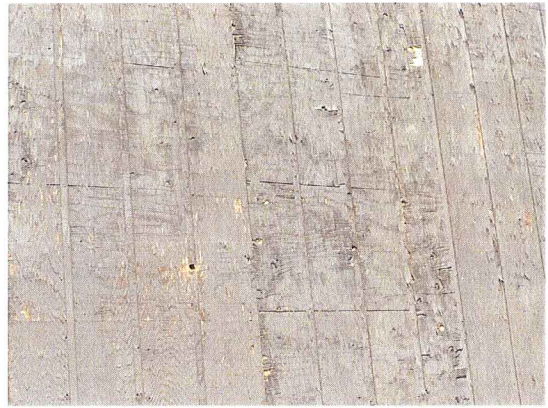
Deteriorated Wood Siding With a Hole 2355-2353 Allied Dr April 10, 2006
