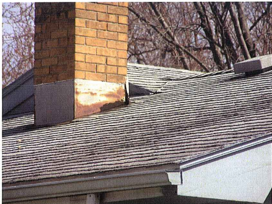
Deteriorated Shingles, Rusted Flashing 4714-4718 Crescent Dr April 10, 2006
