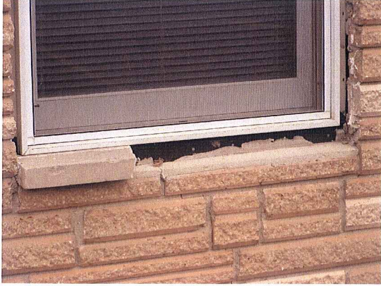
Sill Missing 2306-2302 Allied Dr March 30, 2006
