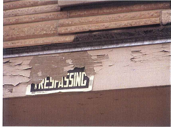
Deteriorated Fascia 2102 Rosenberry March 30, 2006
