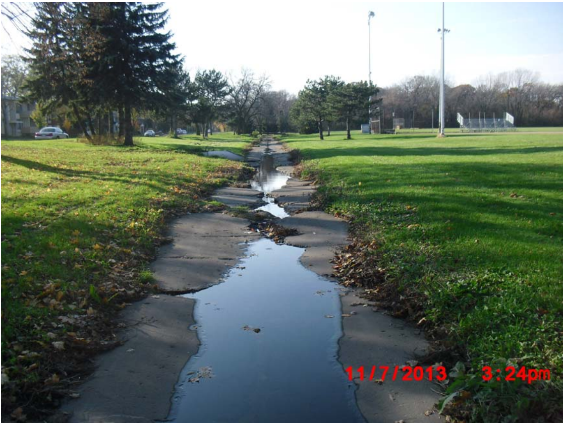
Photograph 5: Existing conditions of the channel. The concrete channel shows significant degradation along Trailsway. Cunette replacement will extend to the wooded area in the background of the photo.
