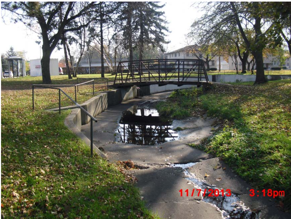
Photograph 3: Existing conditions of the channel. Degraded concrete and sediment deposition are both visible in this photo, which was taken at the 90 degree turn at Sherman Avenue and Trailway intersection.
