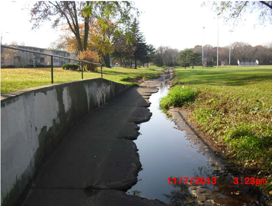
Photograph 4: Existing conditions of the channel. The concrete channel shows significant degradation along Trailsway.
