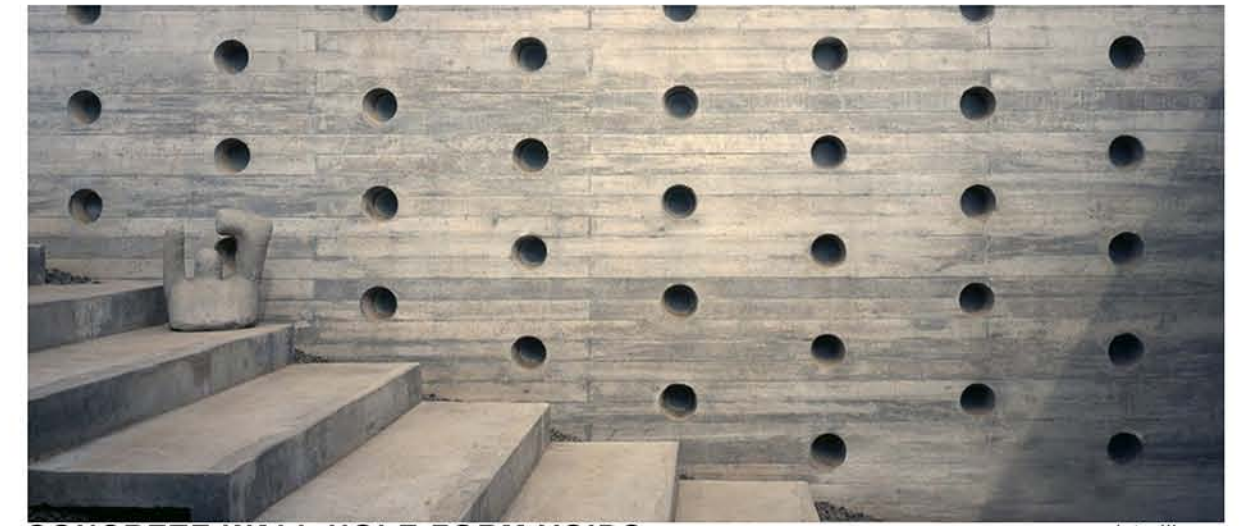
CONCRETE WALL HOLE FORM VOIDS
