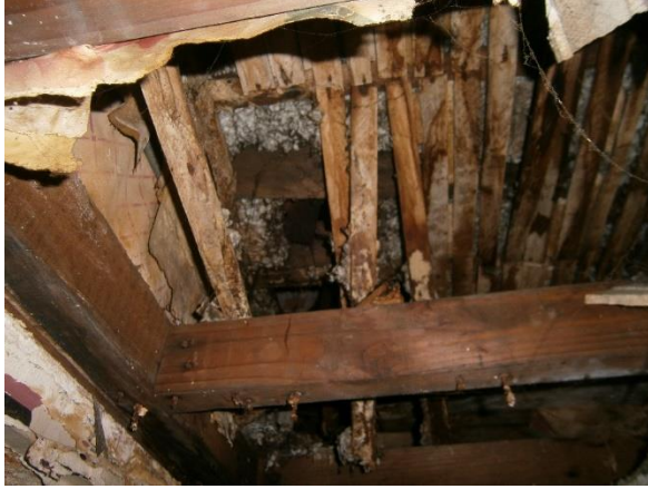
View of deteriorated ceilings and roof in second floor of 510.
