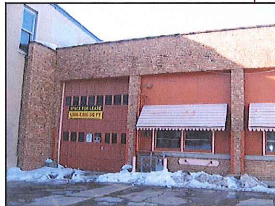
OVERHEAD GARAGE DOOR AND ADJACENT ORIGINAL DOOR OPENING INFILLED WITH WOOD WALLS AND WOOD FRAMED WINDOWS
