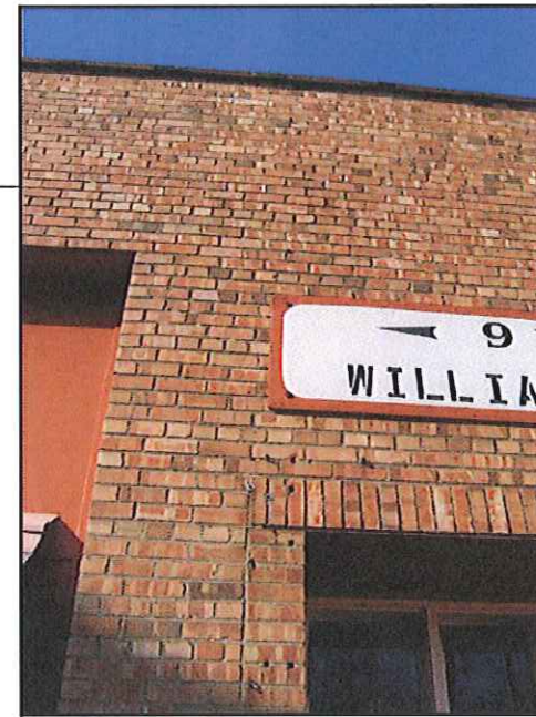
DETAIL IMAGE SHOWING EXISTING WALL MOUNTED SIGNAGE AND CONDITION OF BRICK AND ROOF COPING
