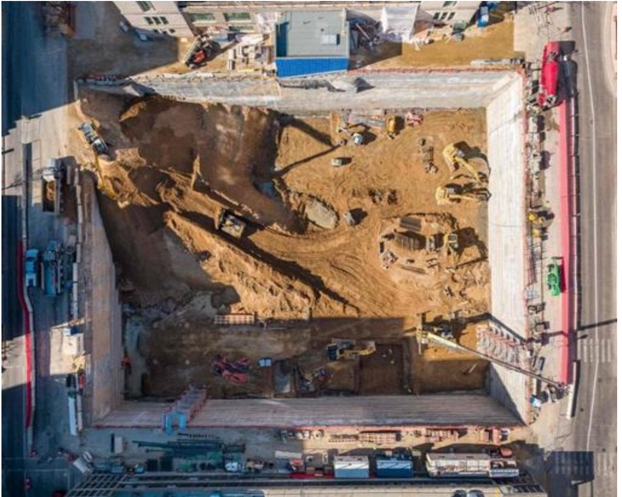
An image of the excavation from above. The Madison Municipal Building Annex is at the top of the picture.
