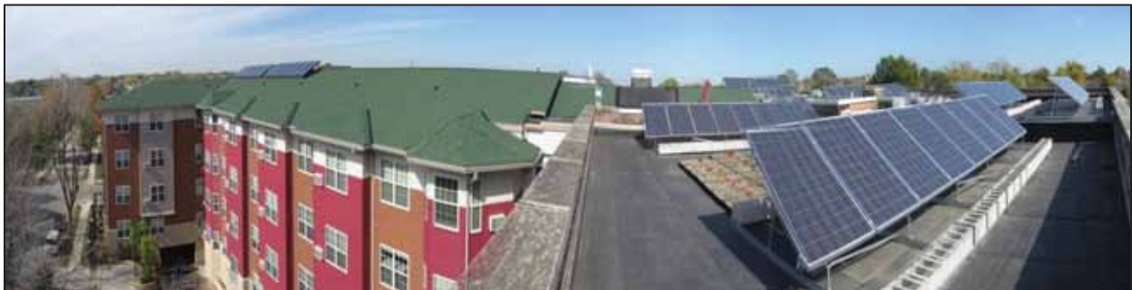
Solar Panels at Dr. Wesley Scott Senior Living—Milwaukee, WI
